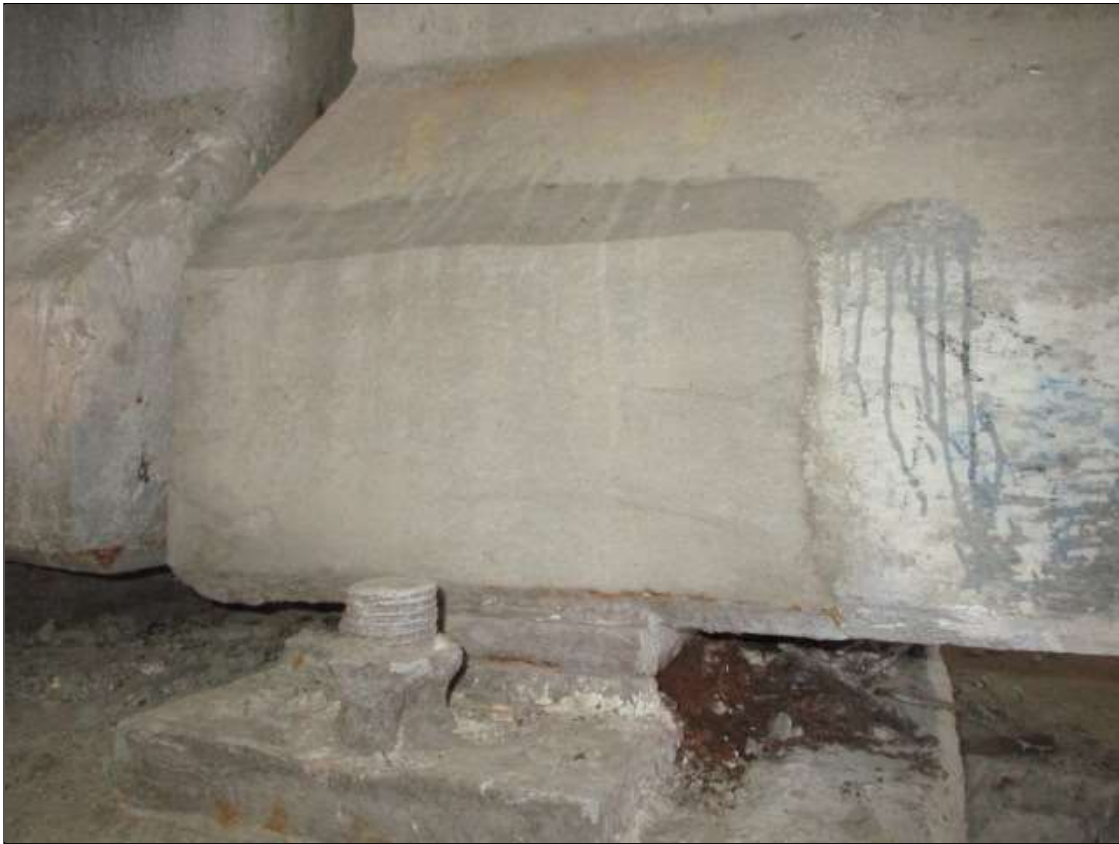
Span 51 Beam 2: 12" LONG X 10" TALL NEW REPAIR TO BOTTOM RIGHT FLANGE AT BENT 50
