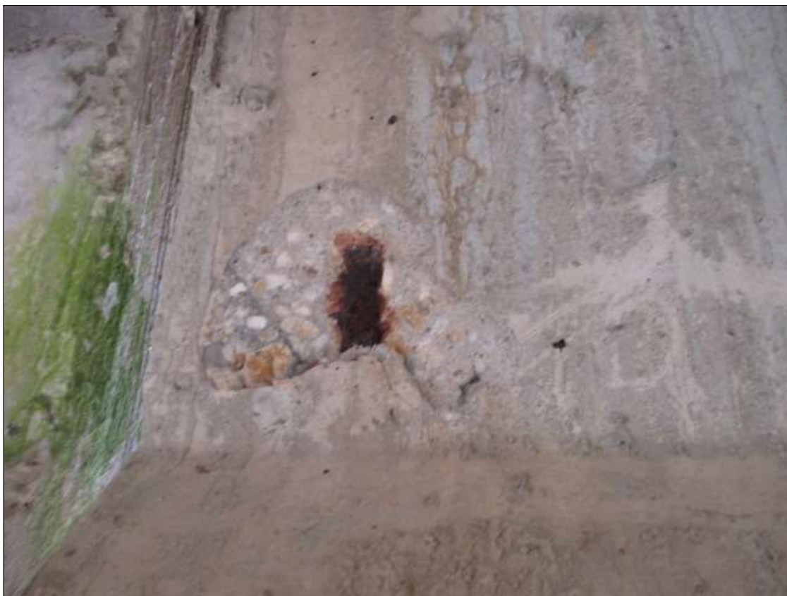
Span 53 Beam 1: SPAN 53 BEAM 1 RIGHT WEB OVER BENT 52. HAS A CRACK/SPALL AND DELAMINATED AREA WITH 1 REBAR VISIBLE. AREA IS: 4" x 5" x 1/2" DEEP. No section loss noted.
