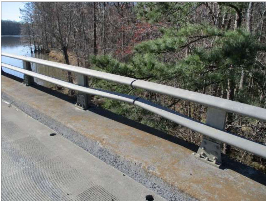
Span 70 Left Bridge Rail: SPAN 70 LEFT RAIL IS BENT UPWARD 3" BETWEEN RAIL POST 4 AND 5.
