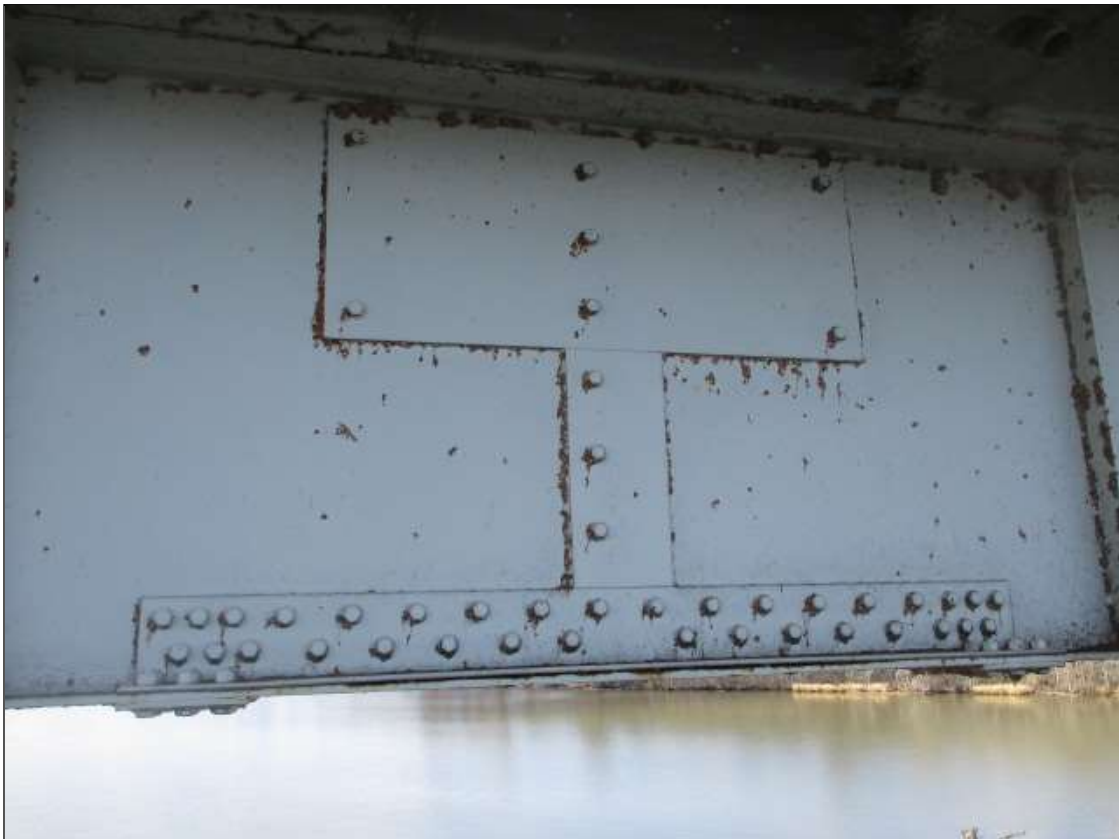
5' LONG X FULL WIDTH REPAIR TO BOTTOM FLANGE AND FULL HEIGHT X UP TO 3' LONG REPAIR TO WEB OF GIRDER 4 SPAN 18 BETWEEN SPLICES
