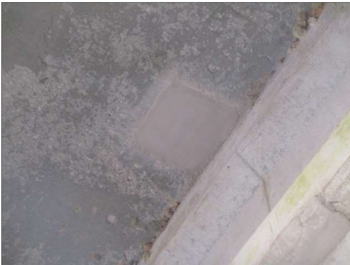
Span 1 Deck: 12" X 12" NEW REPAIR TO UNDERSIDE IN BAY 1 AT 25' FROM END BENT 1 ADJACENT TO GIRDEF 2
