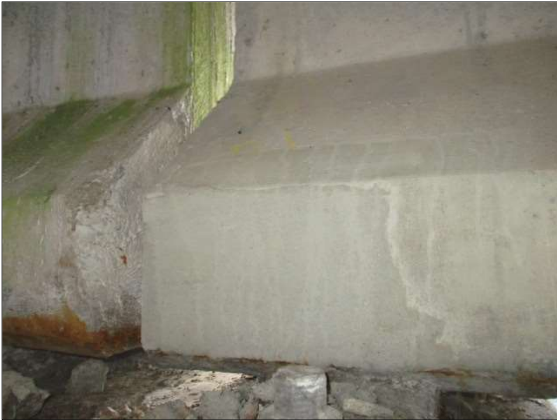
Span 51 Beam 1: 10" LONG X 8" TALL NEW REPAIR TO BOTTOM RIGHT FLANGE AT BENT 50
