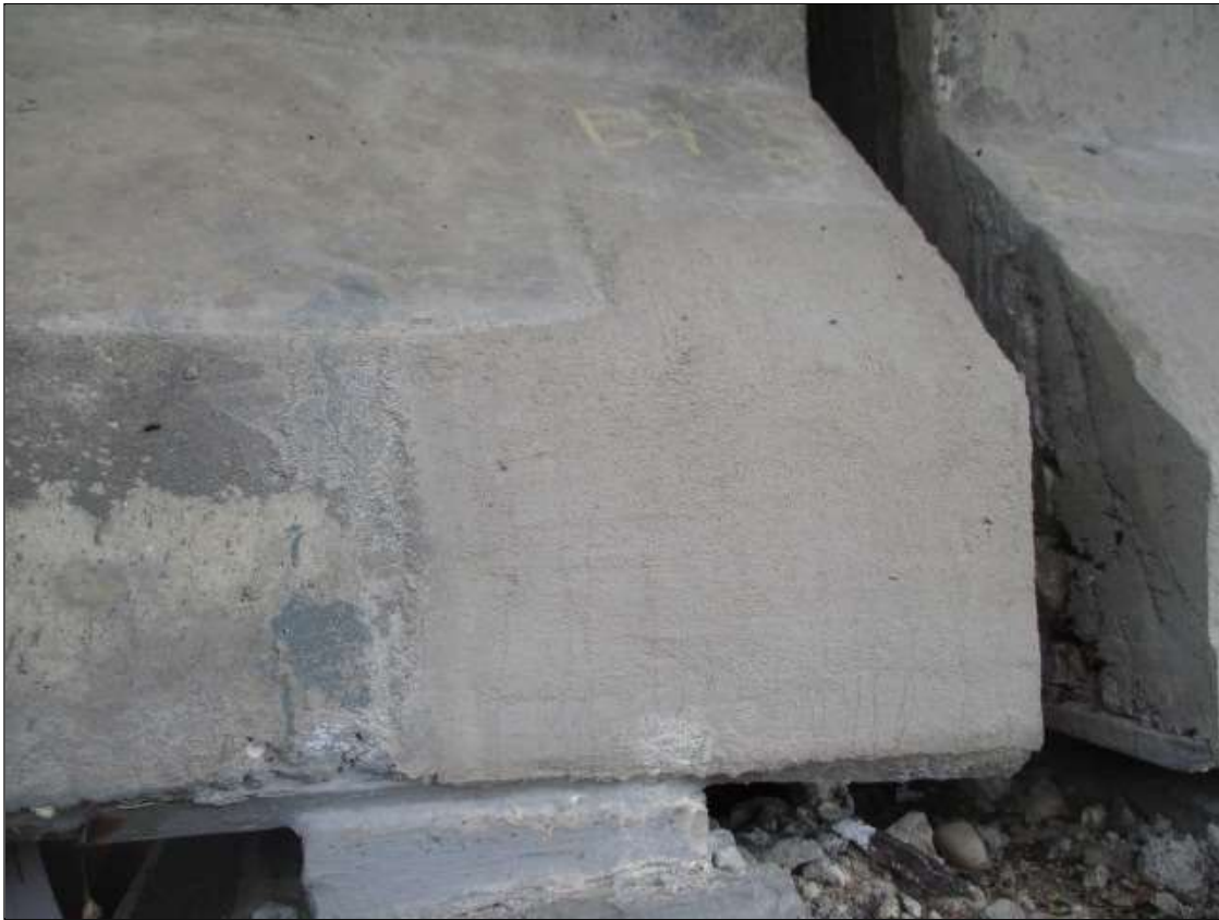
Span 6 Beam 1: 12" LONG X 15" TALL NEW PATCH ON BOTTOM LEFT FLANGE AT BENT 5
