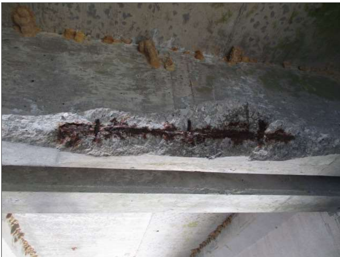
Span 82 Deck: 5' WIDE X 12" TALL X 6" DEEP SPALL WITH EXPOSED REBAR WITH NO SECTION LOSS IN BAY DIAPHRAGM OVER BENT 81
