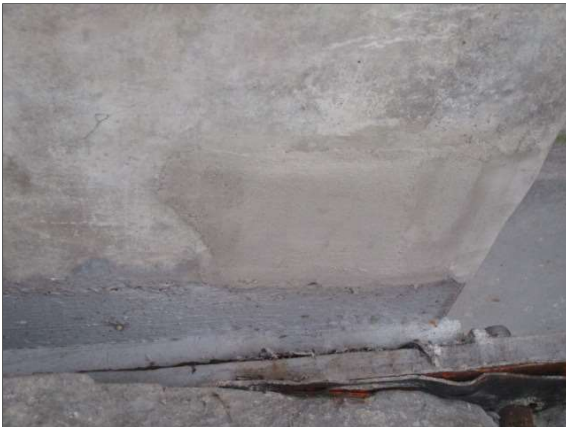
Span 6 Beam 3: 6" LONG X 2" WIDE NEW PATCH ON UNDERSIDE OF BOTTOM FLANGE AT BENT 6
