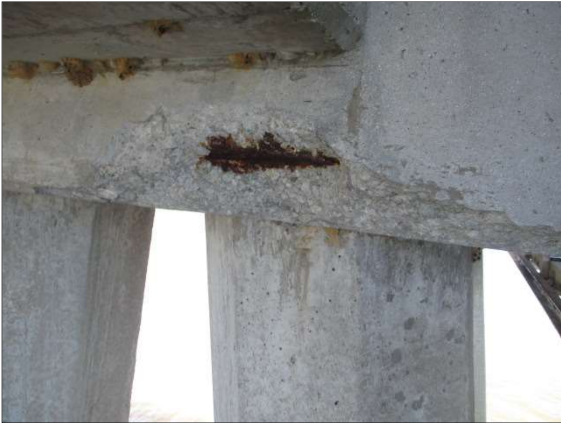
Bent 82 Cap 1: across East face, spall [32in x 4in x 3in deep] with exposed rusted reinforcing [up to 10% section loss] OVER PILES 5 AND 6
