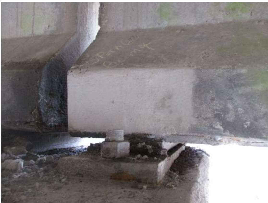
Span 6 Beam 4: 10" LONG X 8" TALL NEW PATCH ON BOTTOM LEFT FLANGE AT BENT 6
