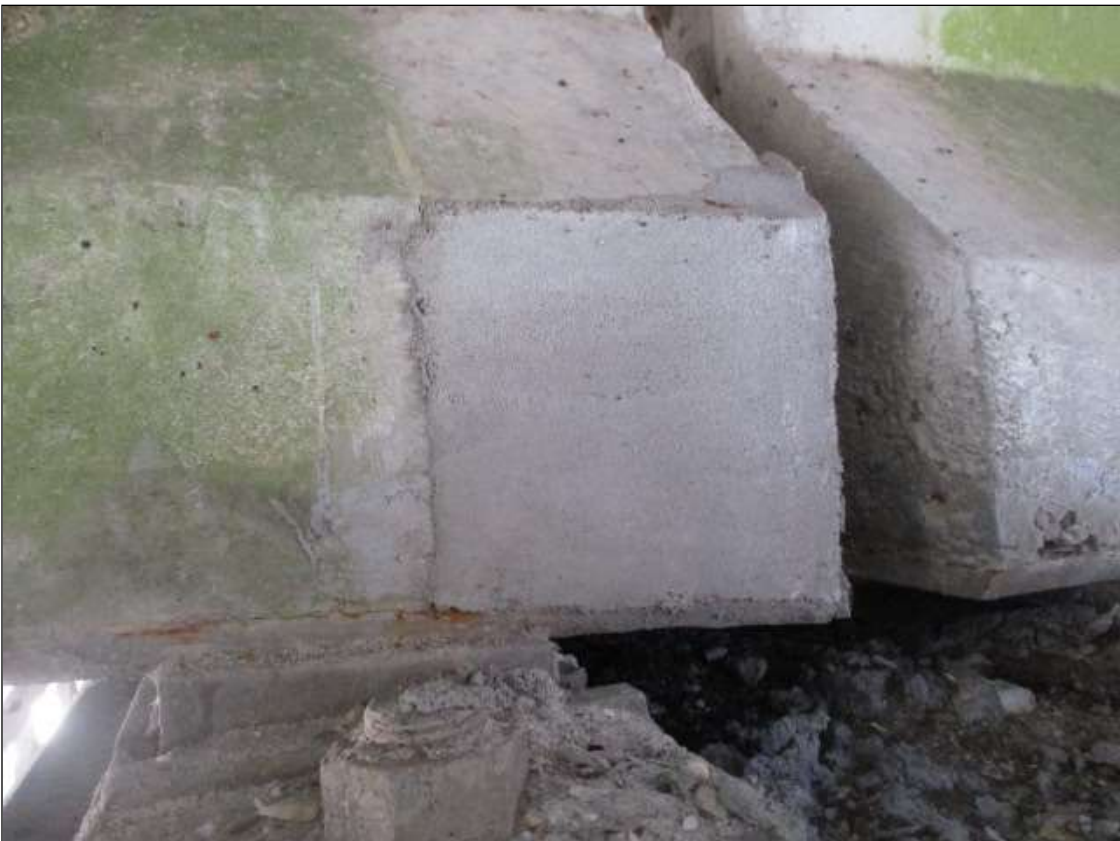
Span 4 Beam 2: 8" LONG X 8" TALL NEW PATCH ON BOTTOM LEFT FLANGE AT BENT 3
