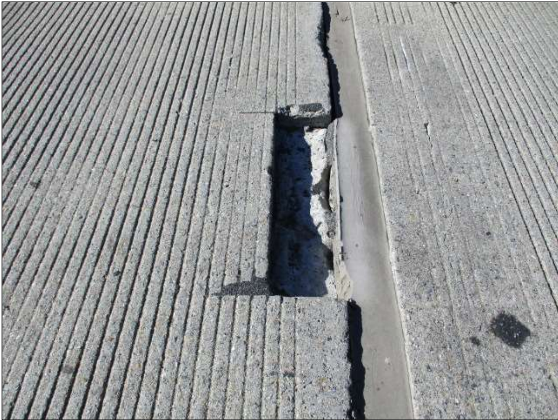
Span 74 Deck: 15" WIDE X 3" LONG X 2" DEEP SPALL IN LEFT LANE AT BENT 74
