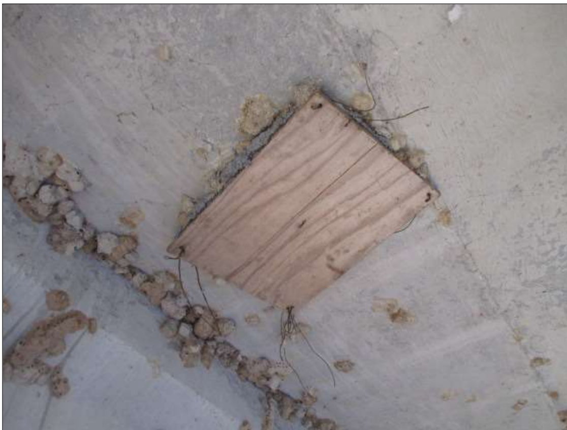
Span 54 Deck: 2' X 2' PATCHED AREA IN BAY 3 AT 30' FROM BENT 53
