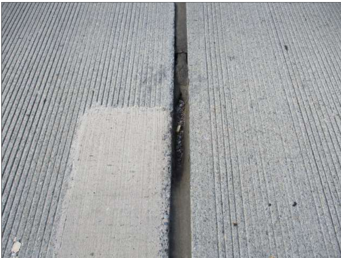
Span 34 Expansion Joint over Bent 33: At centerline, adhesion failure [1ft x full depth]
