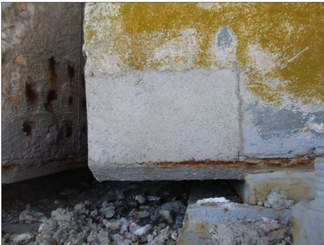
Span 70 Beam 4: 6" LONG X 4" TALL NEW REPAIR TO BOTTOM RIGHT FLANGE AT BENT 69
