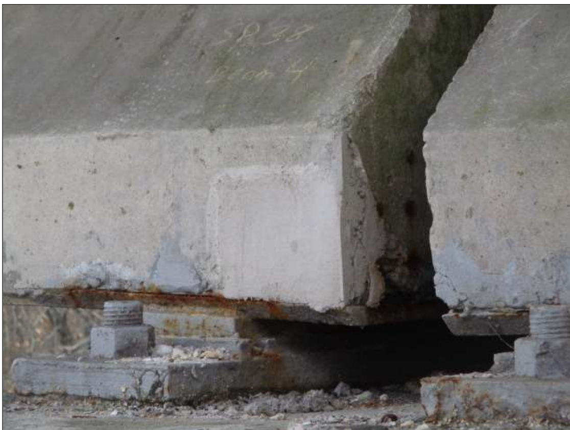
Span 38 Beam 4: 6" LONG X 6" TALL NEW REPAIR TO BOTTOM RIGHT FLANGE AT BENT 38
