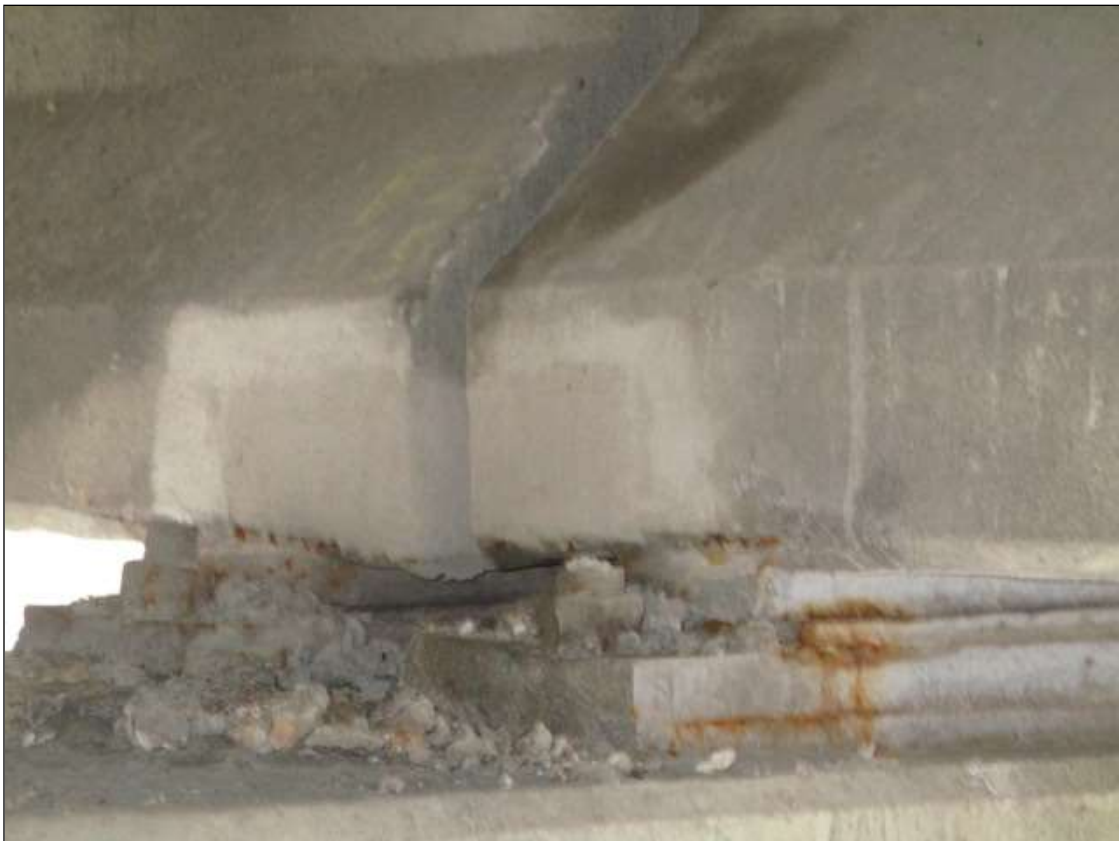
Span 5 Beam 2: 6" LONG X 6" TALL NEW PATCH ON BOTTOM RIGHT FLANGE AT BENT 4
