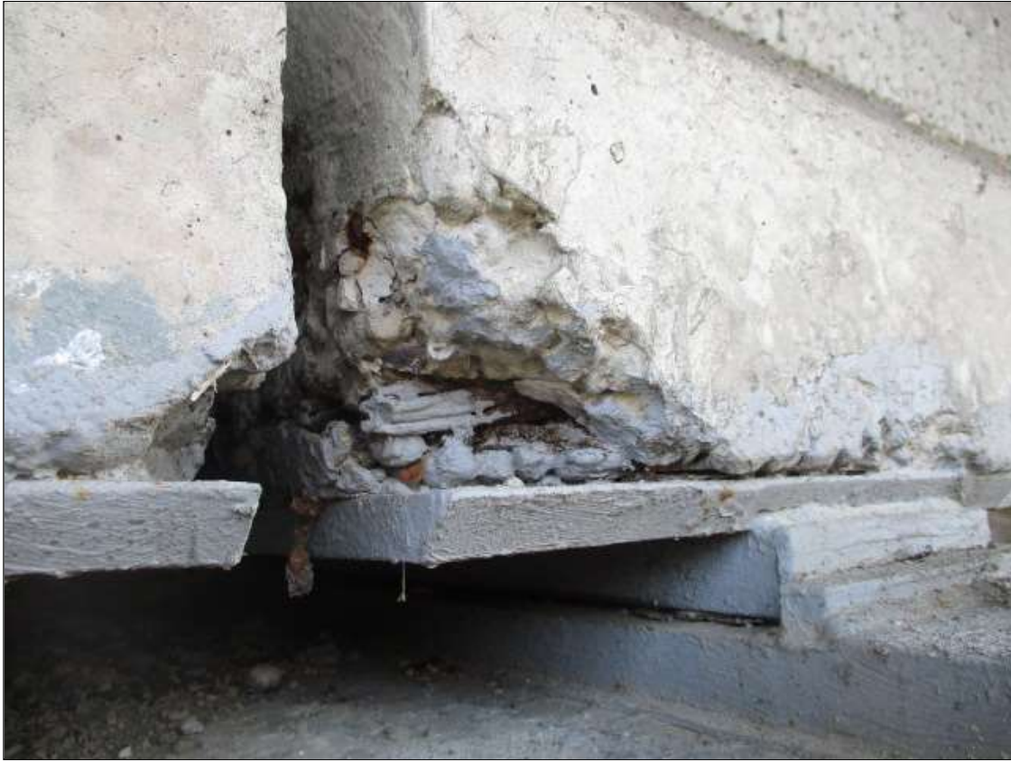
Span 1 Beam 1: West face of bottom flange at bent 1, spall [4in x 3.5in x up to 2in deep] with [1] exposed strand [no section loss]
