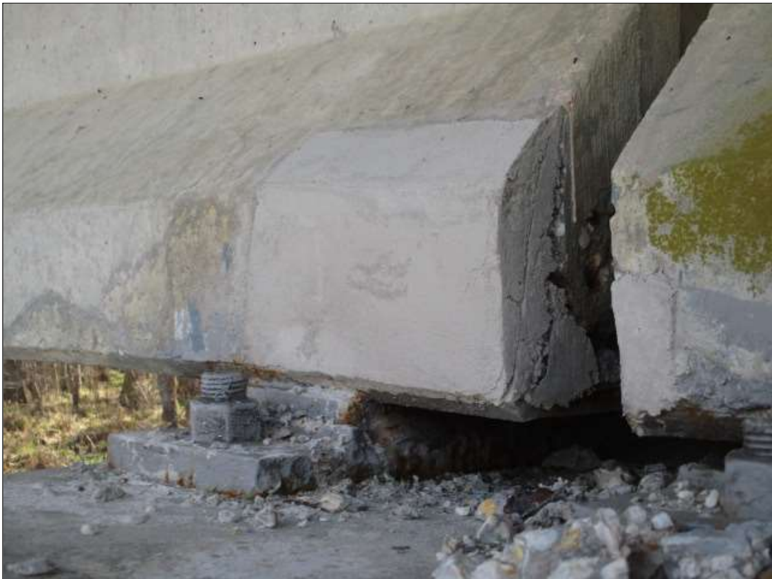
Span 43 Beam 4: 12" LONG X 10" TALL NEW REPAIR TO BOTTOM RIGHT FLANGE AT BENT 43
