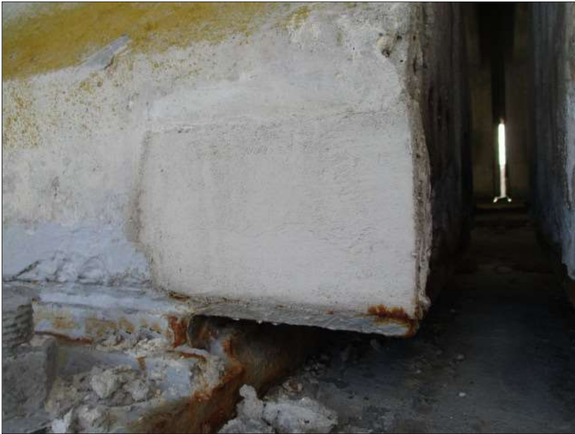
Span 45 Beam 4: 6" LONG X 4" TALL NEW REPAIR TO BOTTOM RIGHT FLANGE AT BENT 45
