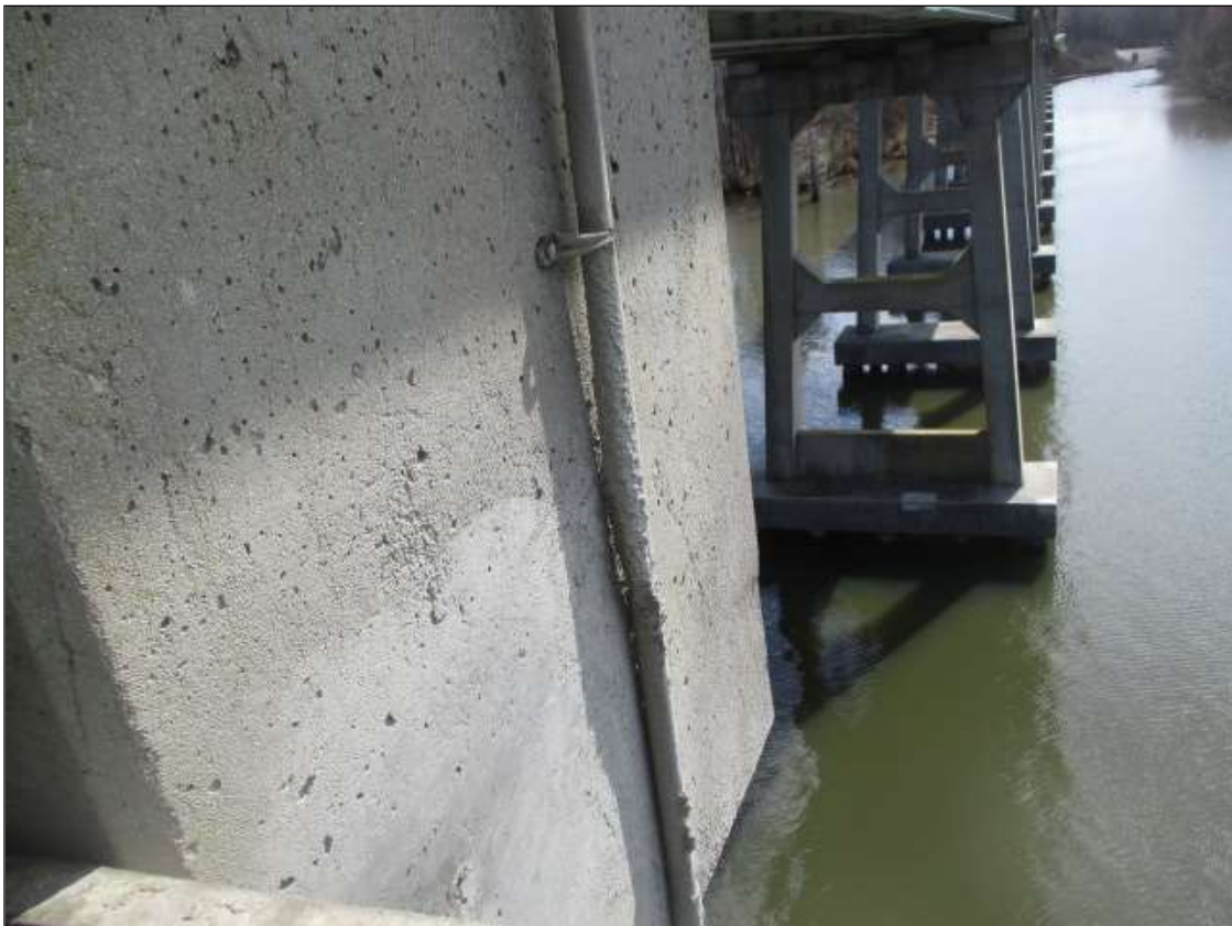
NAVIGATION LIGHT UTILITY ALONG BENT 17 CAP
