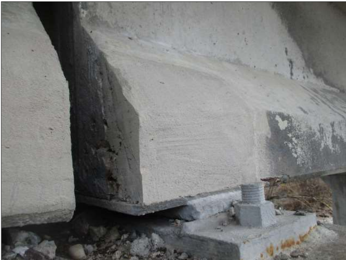
Span 5 Beam 1: 12" LONG X 15" TALL NEW PATCH ON BOTTOM LEFT FLANGE AT BENT 5
