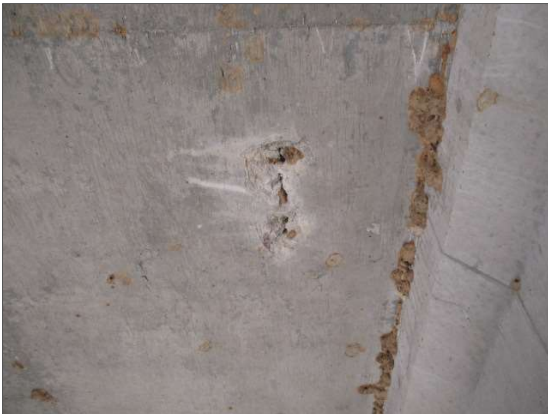
Span 49 Deck: 12" LONG X 6" WIDE X 1" DEEP SPALL IN BAY 2 AT 30' FROM BENT 48
