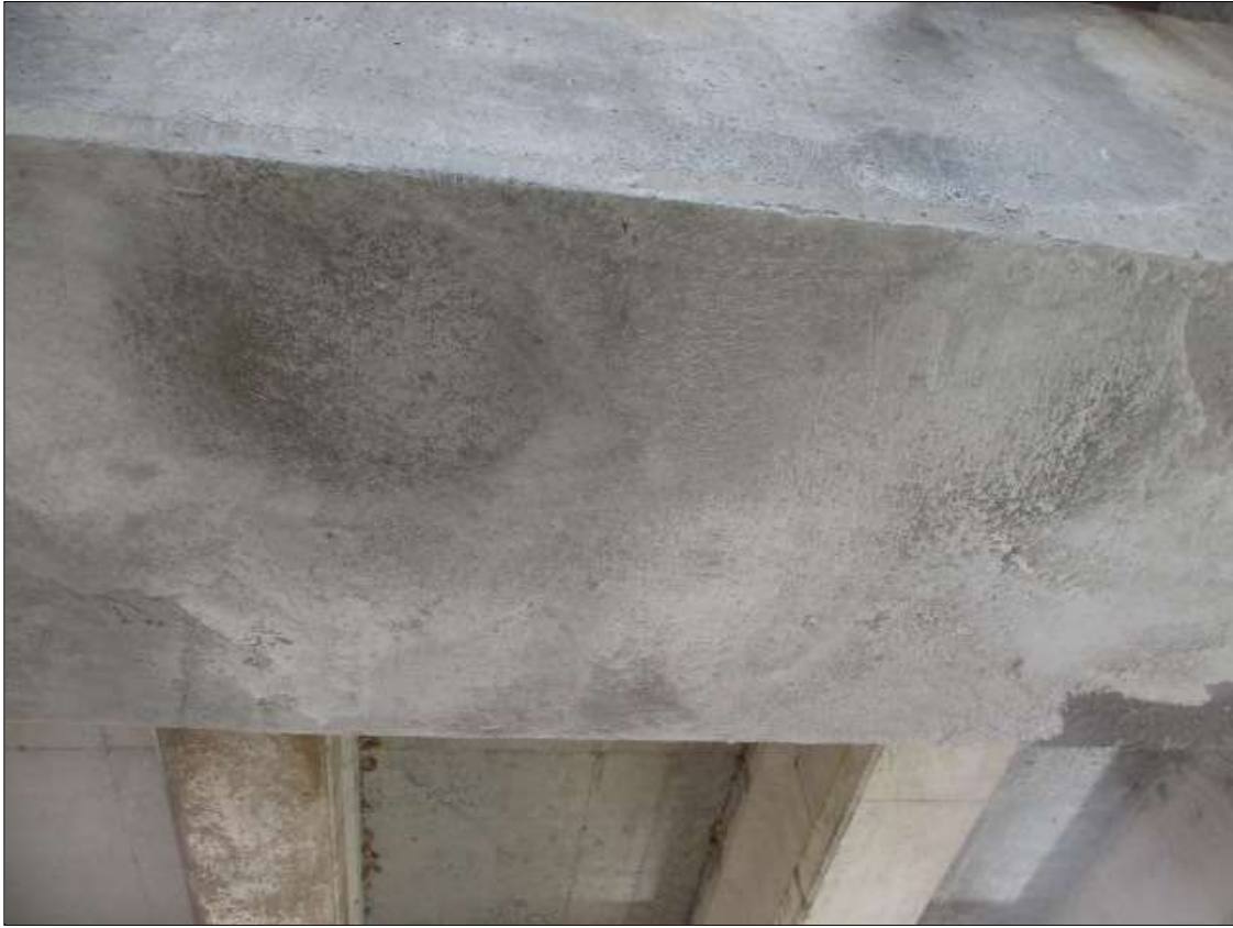
Bent 10 Cap 1: 5' LONG X FULL WIDTH NEW REPAIR TO UNDERSIDE OF CAP
