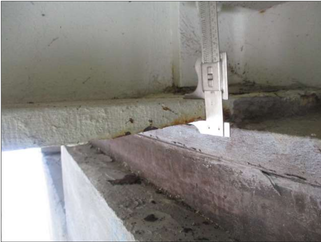
Span 17 Beam 3: PAR: bottom left flange at bent 16, active corrosion with section loss [5in x in x 3/4in avg rem]
