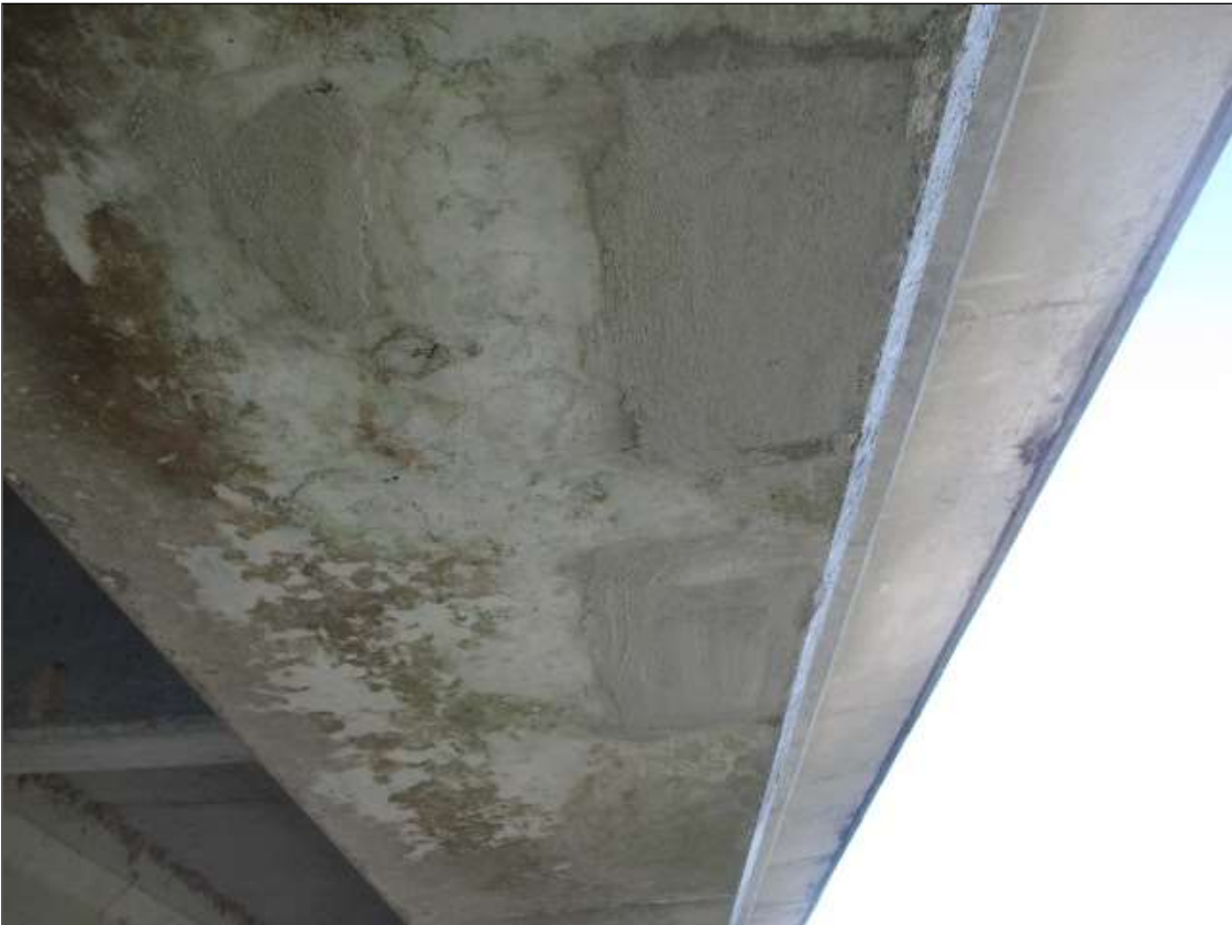
Span 66 Beam 4: 2 - 10" LONG X 6" WIDE NEW PATCHED AREAS ON UNDERSIDE OF BOTTOM FLANGE AT 23' FROM BENT 66
