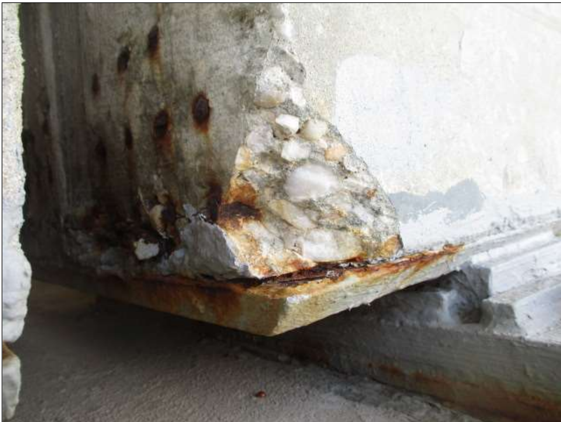
Span 23 Beam 1: West face of bottom flange at bent 23, spall [4in x 4in x 2in deep] with [1] one exposed rusted strand [no section loss]
