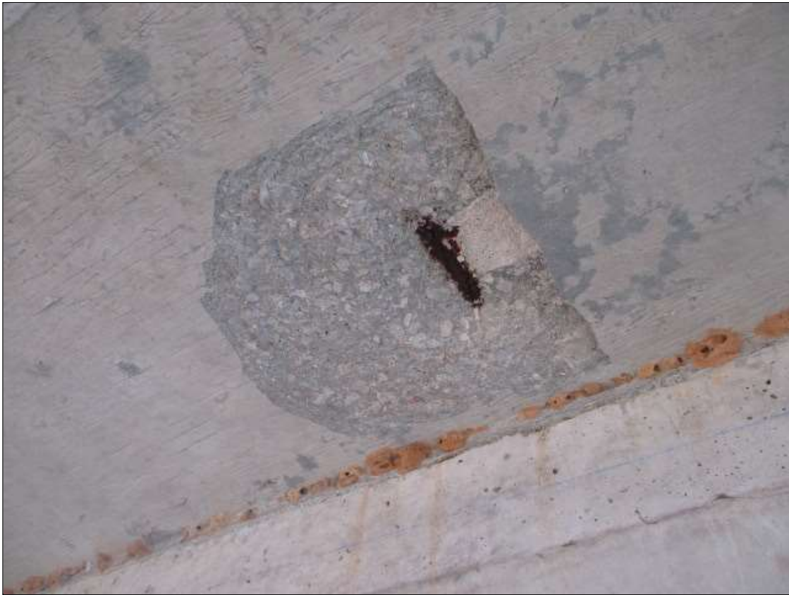
Span 68 Deck: 18" DIAMETER X 1/2" DEEP SPALL WITH EXPOSED REBAR WITH NO SECTION LOSS IN LEFT OVERHANG AT 5' FROM BENT 67
