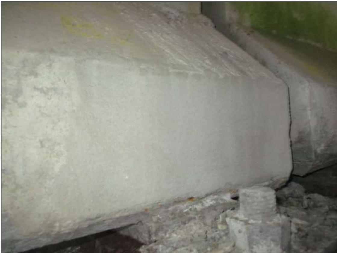
Span 51 Beam 2: 12" LONG X 8" TALL NEW REPAIR TO BOTTOM LEFT FLANGE AT BENT 50
