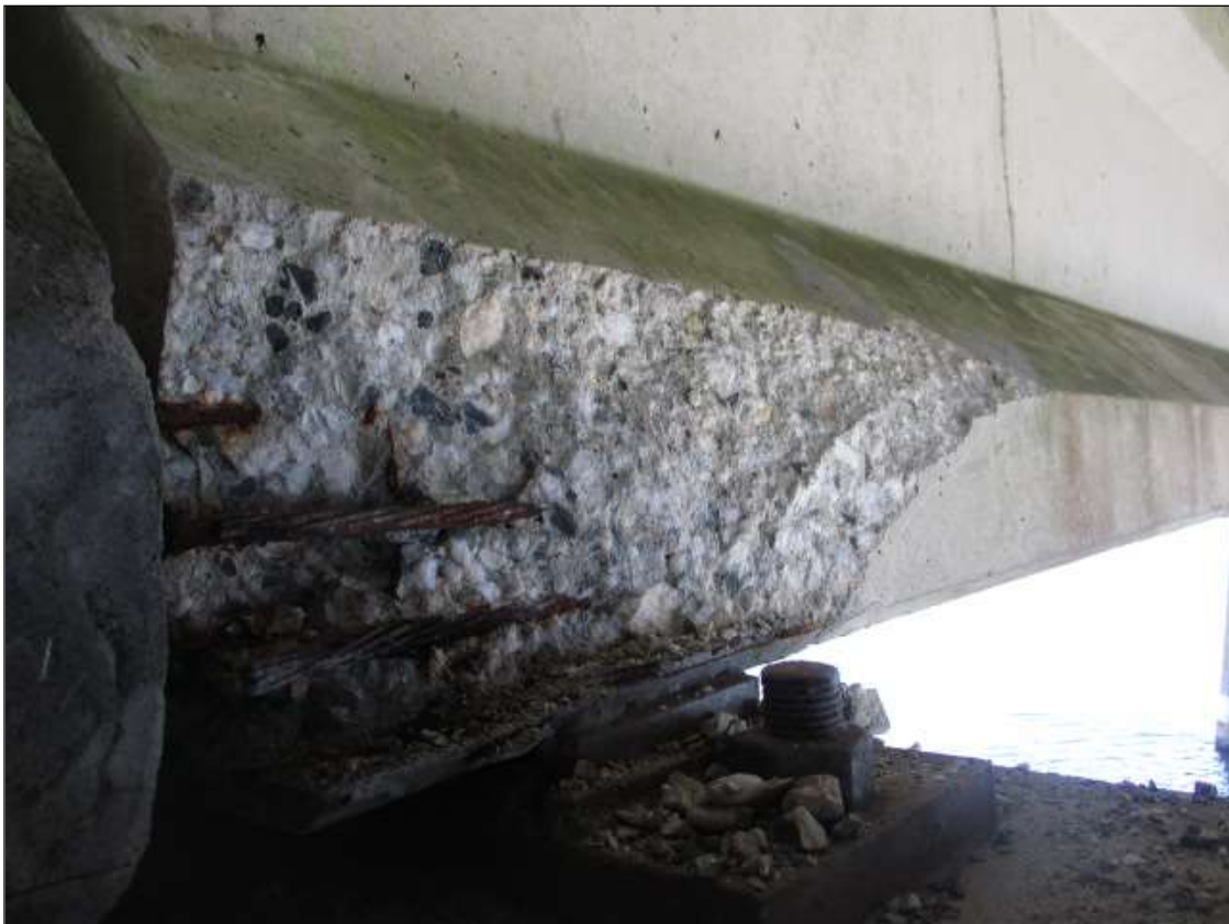
Span 88 Beam 3: PAR: 3' LONG X 10" TALL X 3" DEEP SPALL WITH EXPOSED STRANDS WITH SECTION LOSS ON BOTTOM LEFT FLANGE AT BENT 88
