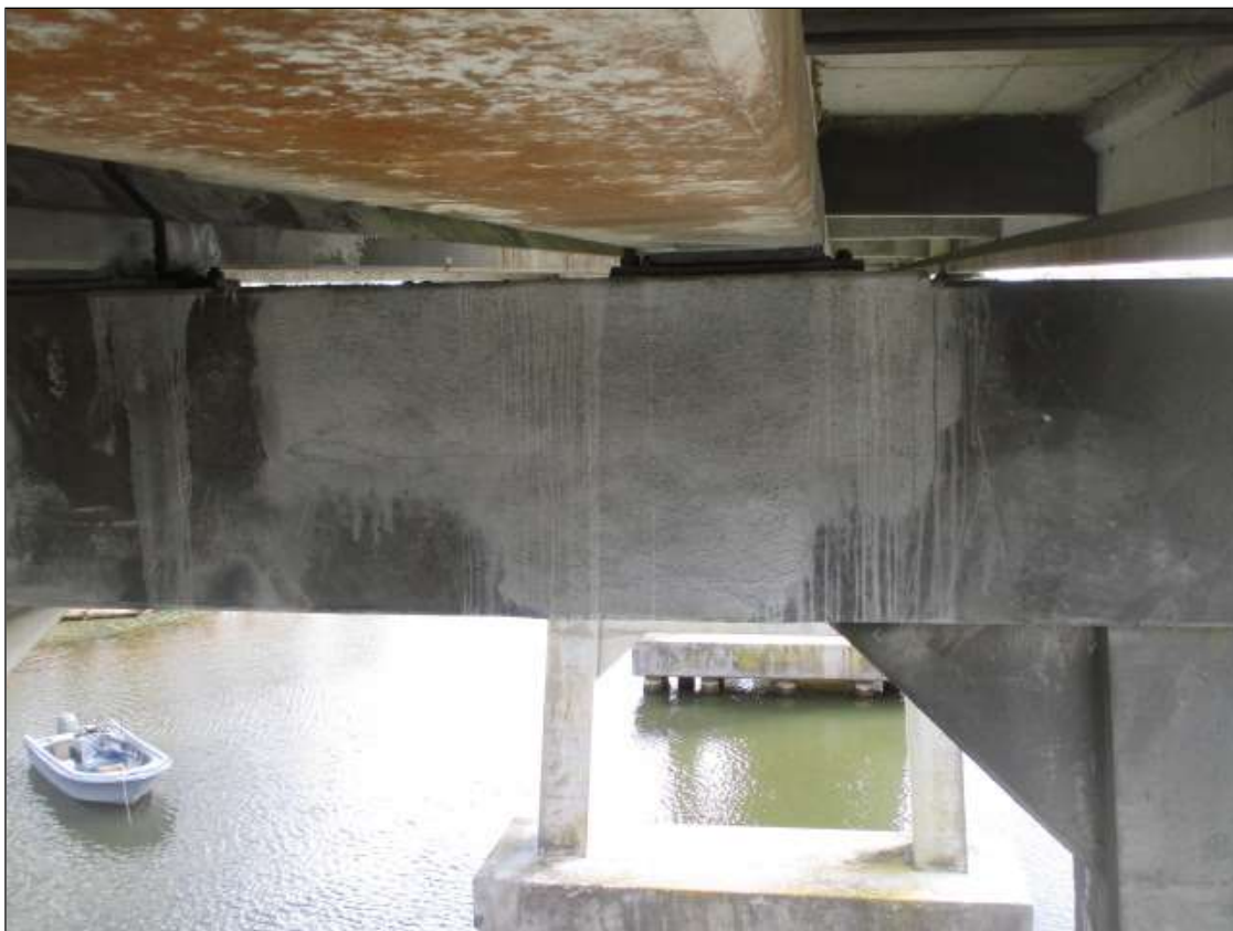
Bent 27 Cap 1: 11' X FULL HEIGHT NEW REPAIR ON NORTH FACE OF BENT 27 CAP UNDER GIRDER 2 AND BAY
