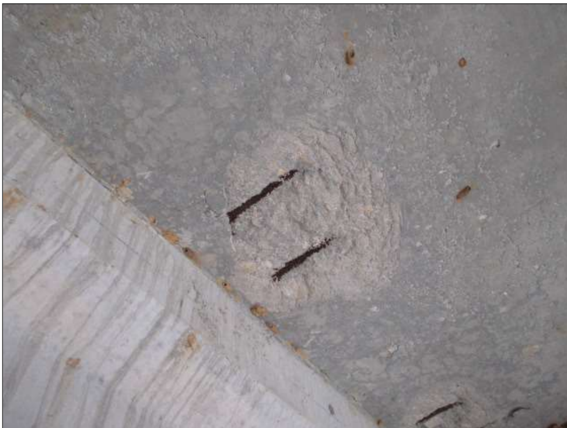
Span 49 Deck: 18" DIAMETER X 1" DEEP SPALL WITH EXPOSED REBAR WITH NO SECTION LOSS IN BAY 3 AT 4' NORTH OF 1ST INTERMEDIATE DIAPHRAGM
