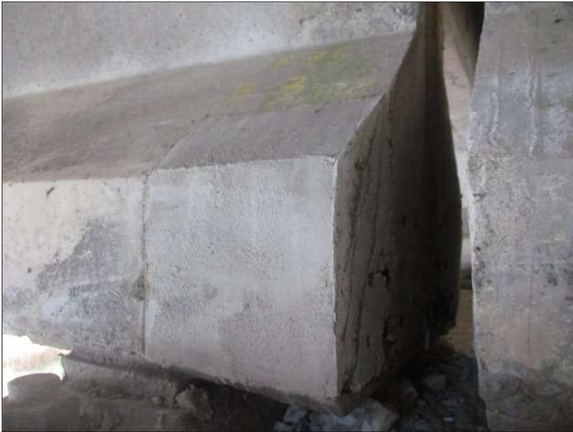
Span 35 Beam 3: 8" LONG X 12" TALL NEW REPAIR TO BOTTOM RIGHT FLANGE AT BENT 35
