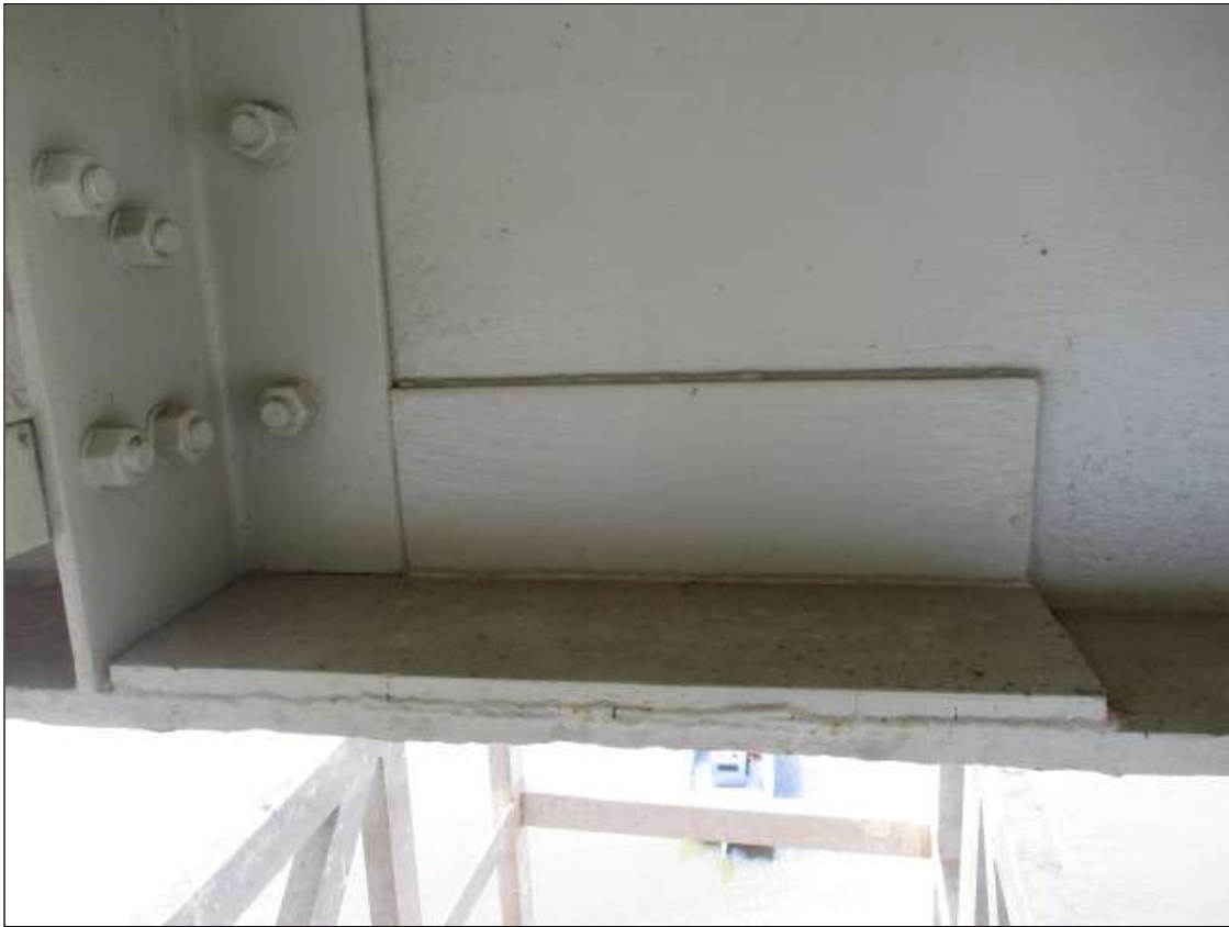
Span 17 Beam 1: SPAN 17 BEAM 1 RIGHT BOTTOM FLANGE AT 3RD CROSS BRACE. HAS A AREA OF SECTION LOSS WITH 5/8" REMAINING. AREA IS: FROM EDGE BACK 7" x 19". Arrested section loss with repair plate in place.
