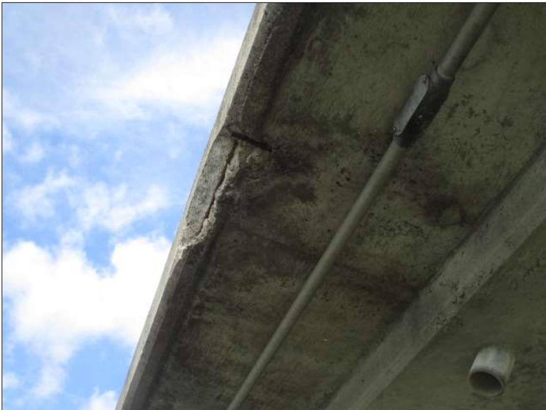
Span 15 Deck: SPAN 15 BOTTOM OF LEFT OVERHANG HAS A SPALLED AREA WITH REBAR EXPOSED. LOCATED 8' FROM BENT 14. AREA IS: 8" x 18" x 1 1/2" DEEP.
