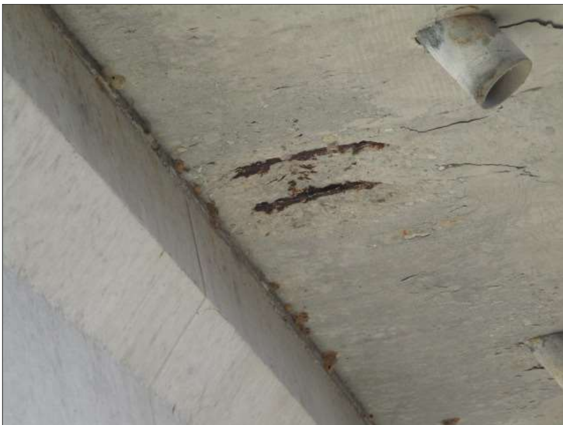
Span 49 Deck: underside of left overhang at 10' from bent 49, spall [18in diameter x 2in deep] with exposed rusted reinforcing [no section loss]
