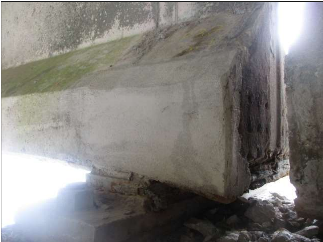
Span 32 Beam 1: 18" LONG X 12" TALL NEW REPAIR TO BOTTOM RIGHT FLANGE AT BENT 32
