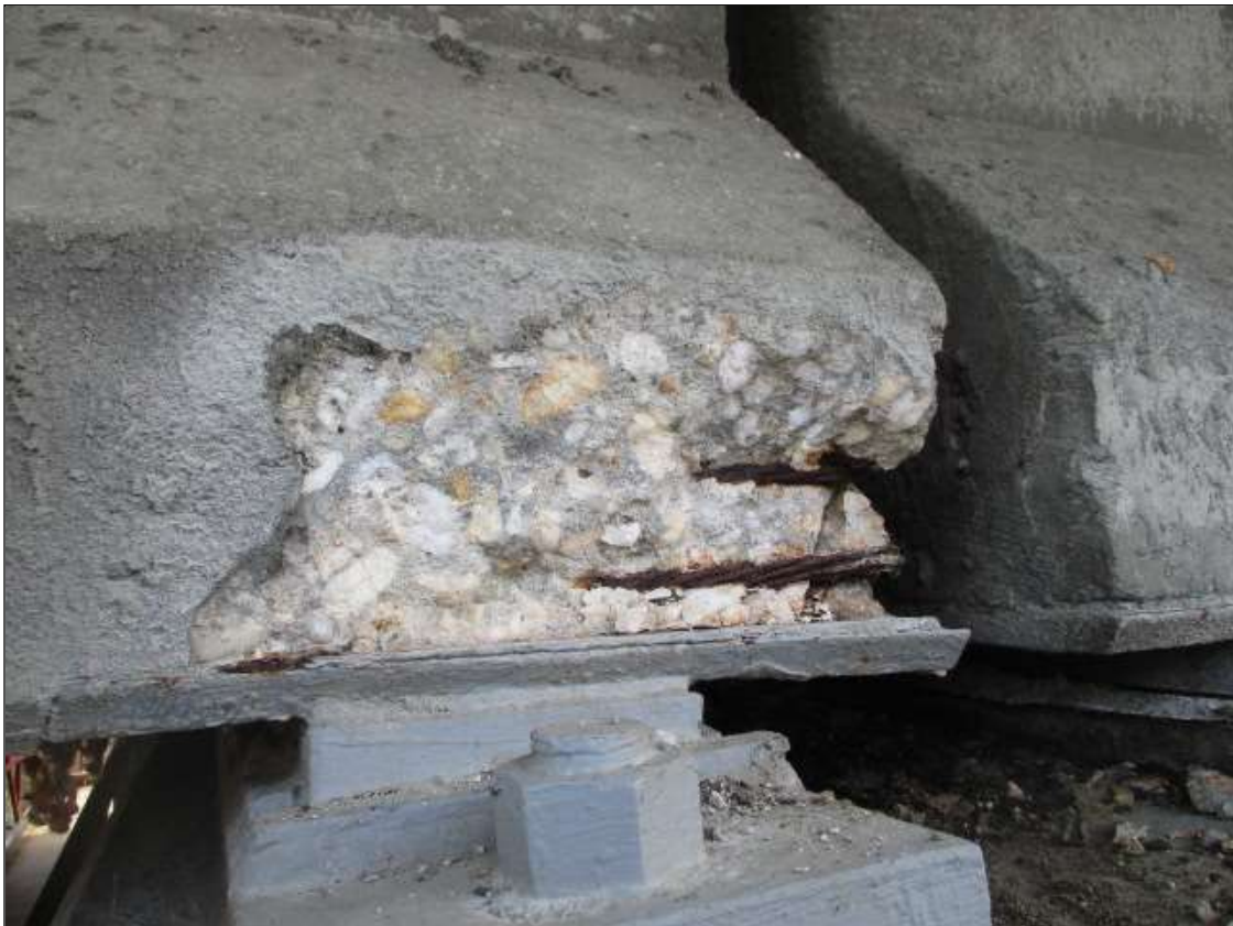
Span 3 Beam 1: [PAR] bottom left flange at bent 2, spall [12in x 8in x 3in deep] with [2] two exposed rusted stirrup [up to 1/16in section loss]
