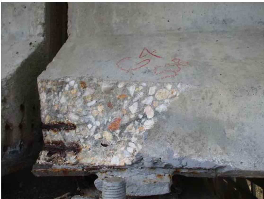
Span 38 Beam 4: PAR: 12" LONG X 8" TALL X 3" DEEP SPALL WITH EXPOSED STRANDS WITH SOME SECTION LOSS ON BOTTOM RIGHT FLANGE AT BENT 37
