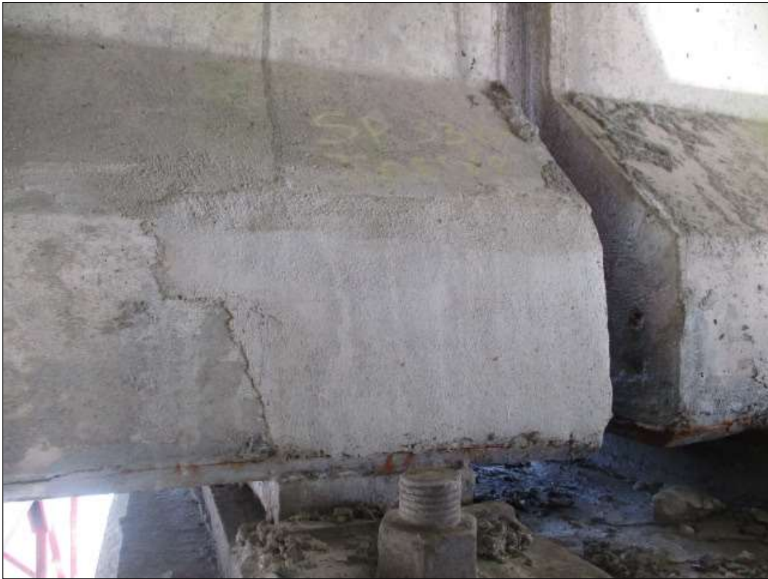
Span 33 Beam 4: 12" LONG X 10" TALL NEW REPAIR TO BOTTOM LEFT FLANGE AT BENT 32
