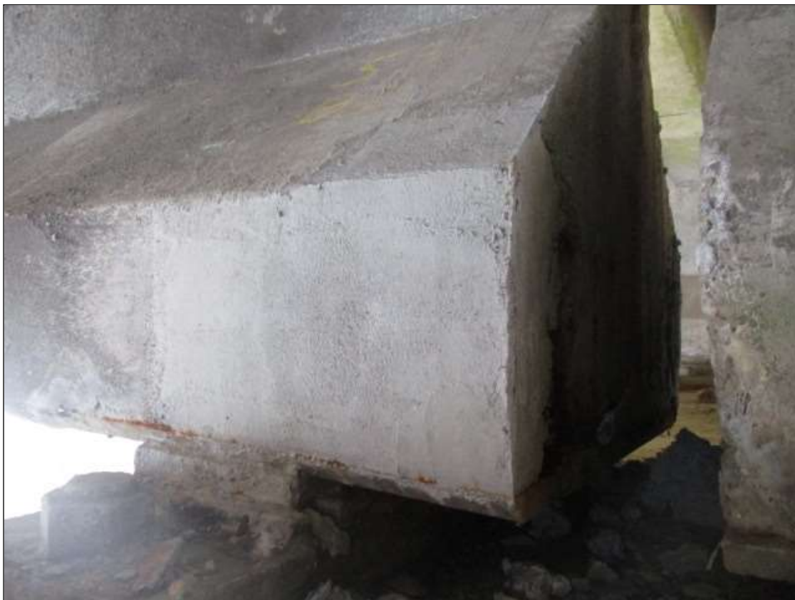
Span 34 Beam 3: 12" LONG X 10" TALL NEW REPAIR TO BOTTOM RIGHT FLANGE AT BENT 34
