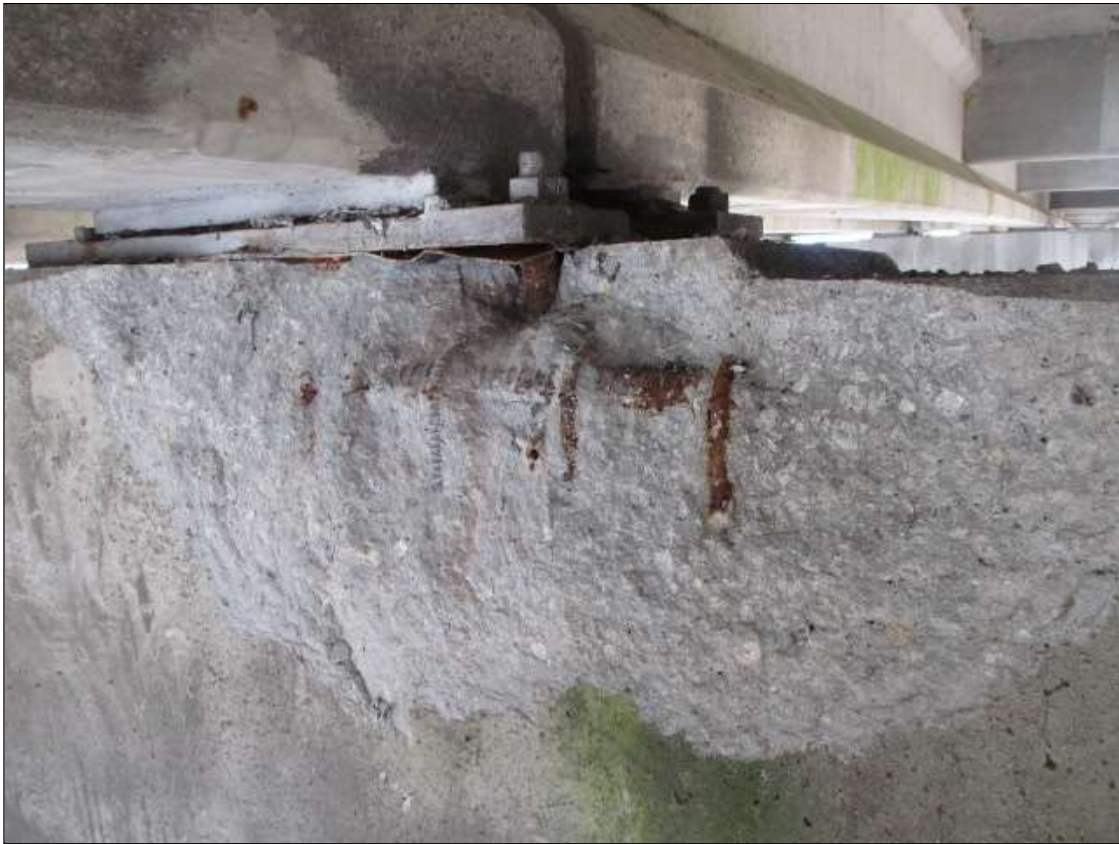
Bent 6 Cap 1: PAR: 4' LONG X 2' TALL X 10" DEEP SPALL WITH EXPOSED REBAR ON SOUTH FACE UNDER GIRDER 3 WITH 18" LONG X 6" DEEP TRIANGULAR AREA OF LOSS OF BEARING
