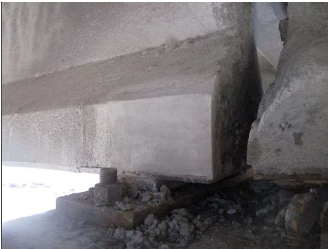
Span 7 Beam 3: 10" LONG X 10" TALL NEW PATCH ON BOTTOM RIGHT FLANGE AT BENT 7
