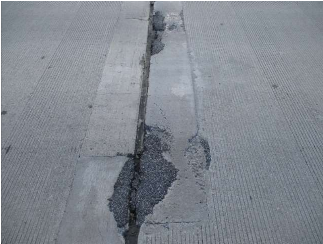
Span 59 Deck: 8' WIDE X 1' LONG CONCRETE AND ASPHALT PATCHED AREA IN NORTH BOUND LANE AT BENT 58
