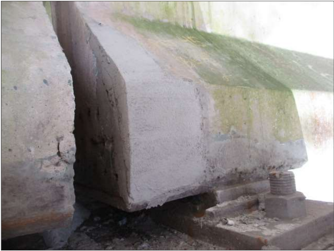
Span 45 Beam 2: 6" LONG X 12" TALL NEW REPAIR TO BOTTOM LEFT FLANGE AT BENT 45
