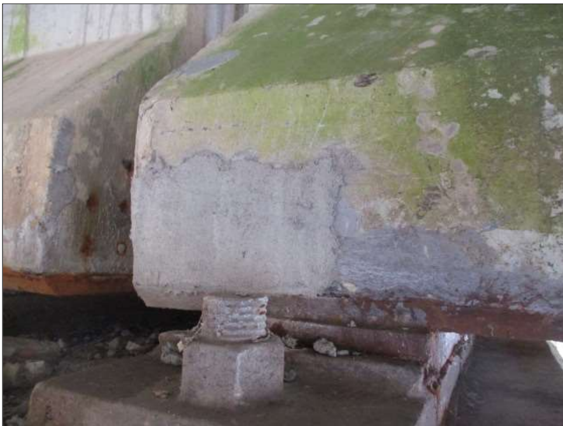
Span 44 Beam 3: 6" LONG X 4" TALL NEW REPAIR TO BOTTOM RIGHT FLANGE AT BENT 43
