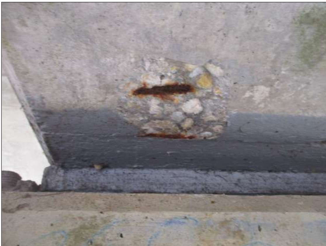
Span 53 Beam 2: underside of bottom flange at near end, spall [4in x 4in x 1/2in deep] with exposed stirrup [no section loss noted]
