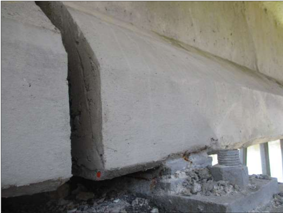
Span 76 Beam 1: 24" LONG X 18" TALL NEW REPAIR TO BOTTOM LEFT FLANGE AT BENT 76
