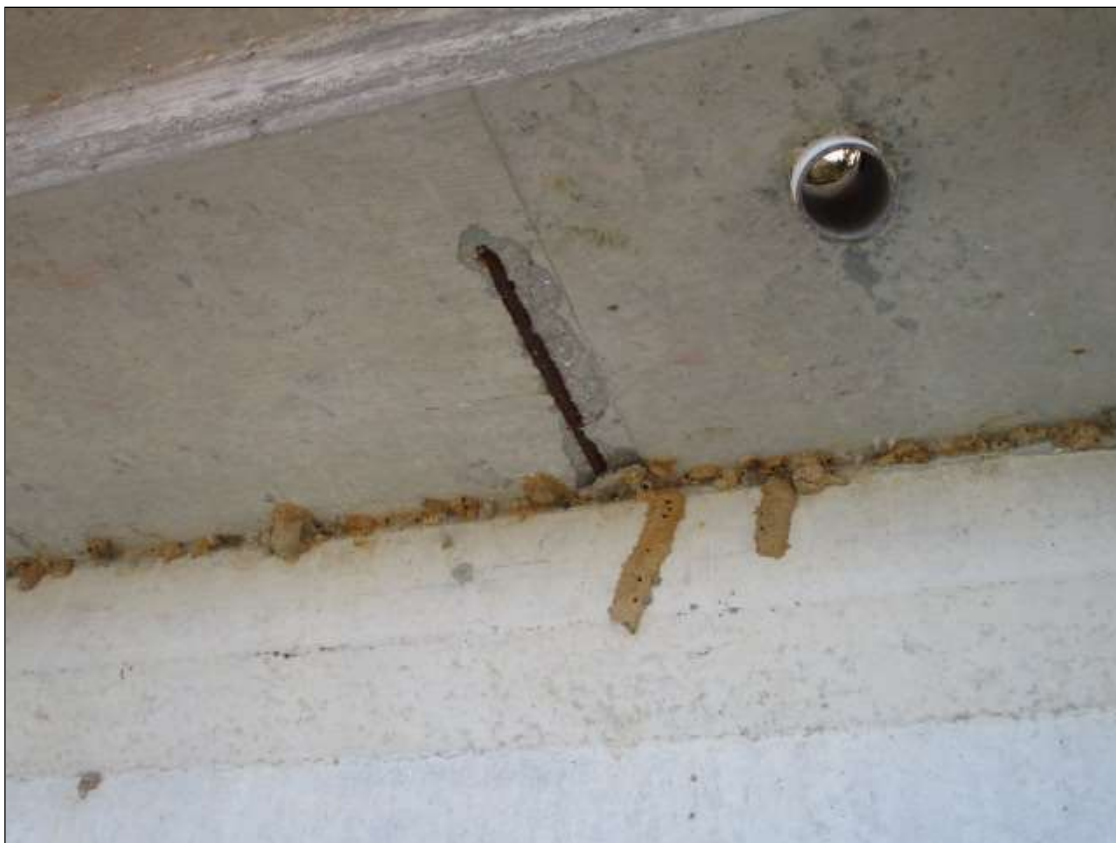
Span 69 Deck: 18" WIDE X 3" LONG X 1/2" DEEP SPALL WITH EXPOSED REBAR WITH NO SECTION LOSS IN RIGHT OVERHANG AT 10' FROM BENT 69
