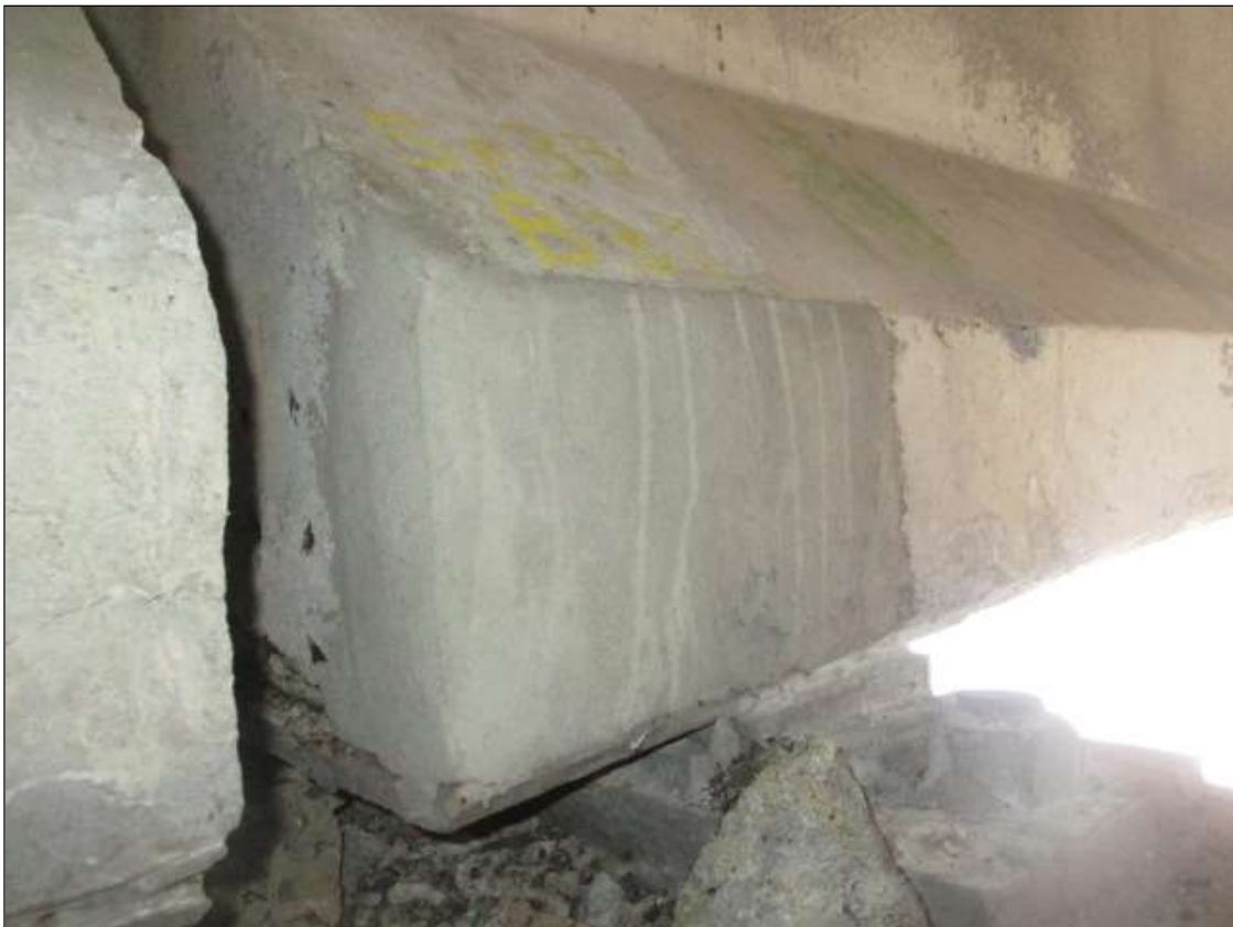
Span 35 Beam 3: 12" LONG X 8" TALL NEW REPAIR TO BOTTOM LEFT FLANGE AT BENT 35
