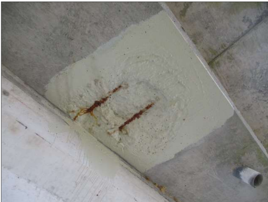
Span 11 Deck: underside of right overhang, spall/failed patch [18in diameter x 2in deep] with exposed rusted reinforcing [up to 10% section loss]
