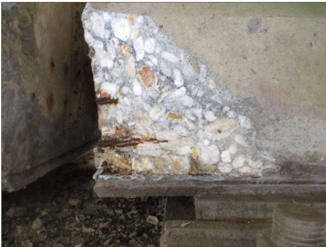
Span 47 Beam 2: PAR: 8" LONG X 8" TALL X 3" DEEP SPALL WITH EXPOSED STRANDS WITH SECTION LOSS ON BOTTOM RIGHT FLANGE AT BENT 46
