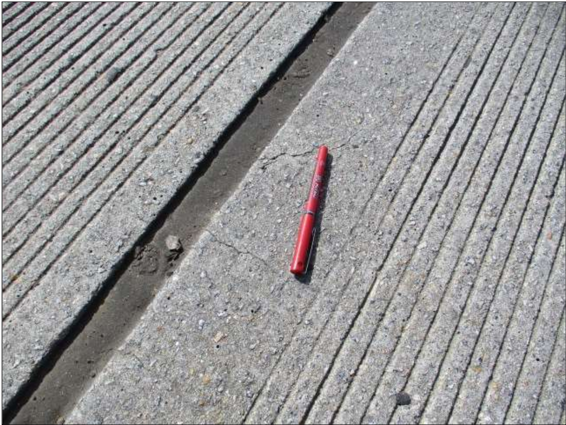
Span 15 Deck: 1/32" LONGITUDINAL CRACKING ALONG JOINTS
