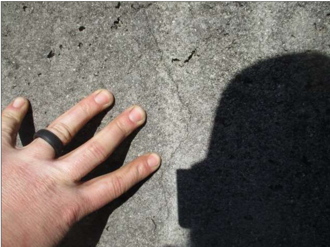
Bent 4 Footing: 1/32" VERTICAL CRACKING ALONG ALL FACES
