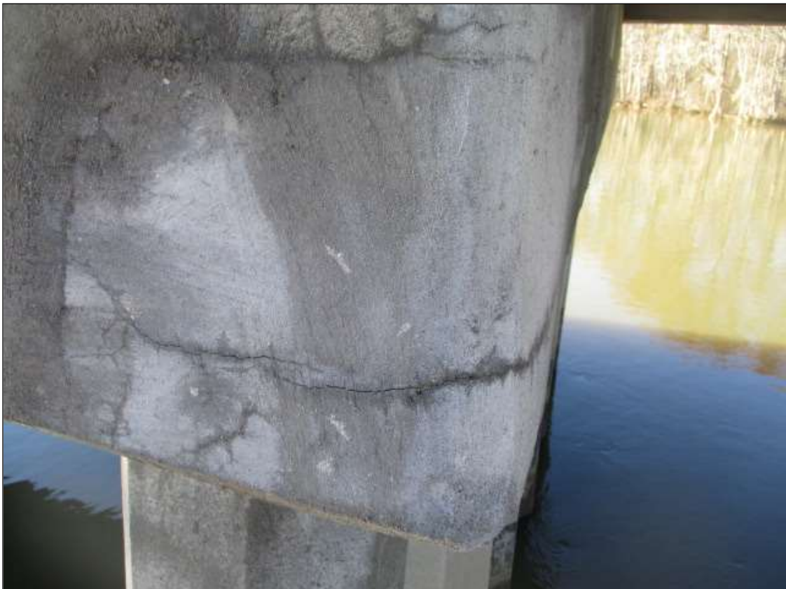
Bent 61 Cap 1: 1/32" HORIZONTAL CRACKING IN PATCHED AREA ON NORTHEAST CORNER
