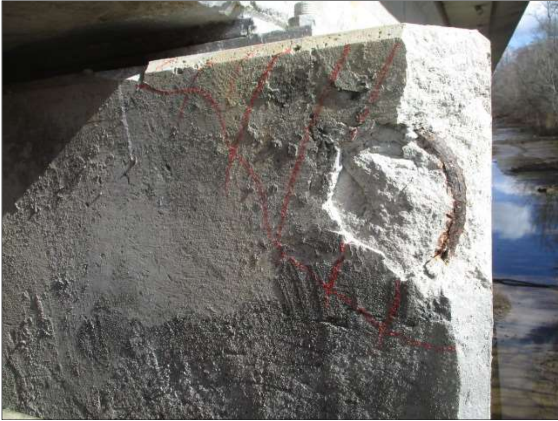
Bent 55 Cap 1: BENT 55 CAP TOP AND NORTH FACE UNDER GIRDER 1. HAS A SPALLED AND DELAMINATED AREA. AREA IS: FROM TOP EDGE BACK 6", FROM TOP EDGE DOWN 10" x 24", TOTAL AREA IS 2.5' LONG X 24" DELAMINATION WITH UP TO 8" DEEP SPALLING WITH EXPOSED REBAR
