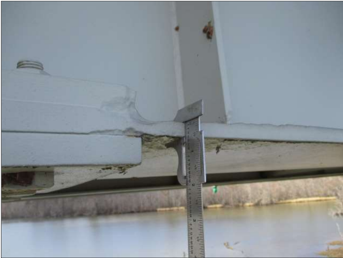
Span 17 Beam 4: PAR: 1/2" REMAINING ON BOTTOM RIGHT FLANGE FOR 3" WIDE X 3" LONG ON NORTH SIDE OF SPLICE NUMBER 1 IN SPAN 18
