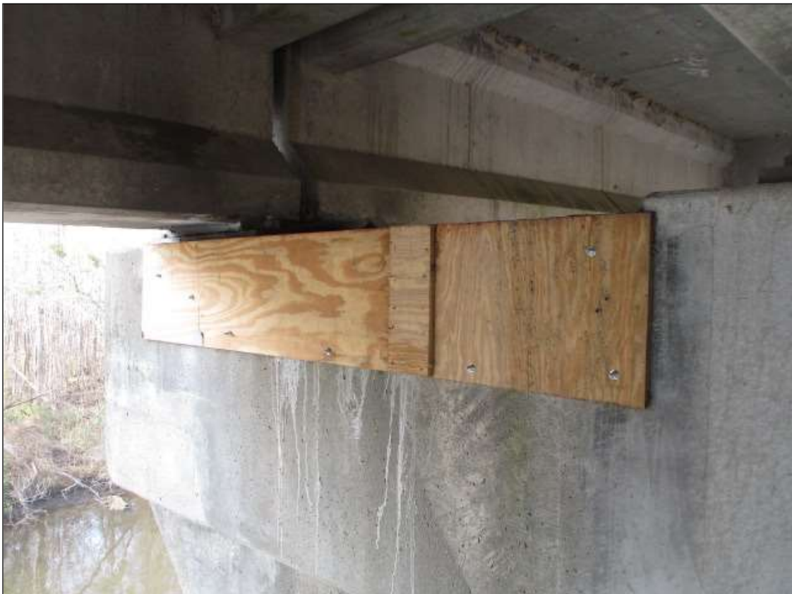
Bent 6 Cap 1: 6' LONG X 12" TALL NEW REPAIR TO SOUTH FACE UNDER BAY 1
