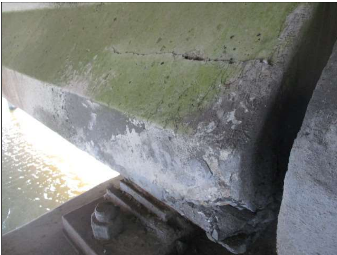
Span 88 Beam 3: SPAN 88 BEAM 3 RIGHT BOTTOM FLANGE OVER BENT 88. DELAMINATED AREA THAT IS 2' LONG X 18" TALL
