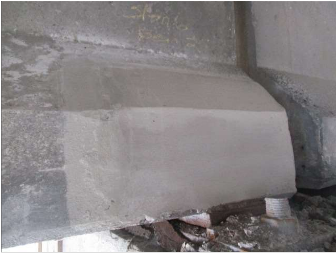
Span 6 Beam 2: 24" LONG X 18" TALL NEW PATCH ON BOTTOM RIGHT FLANGE AT BENT 6
