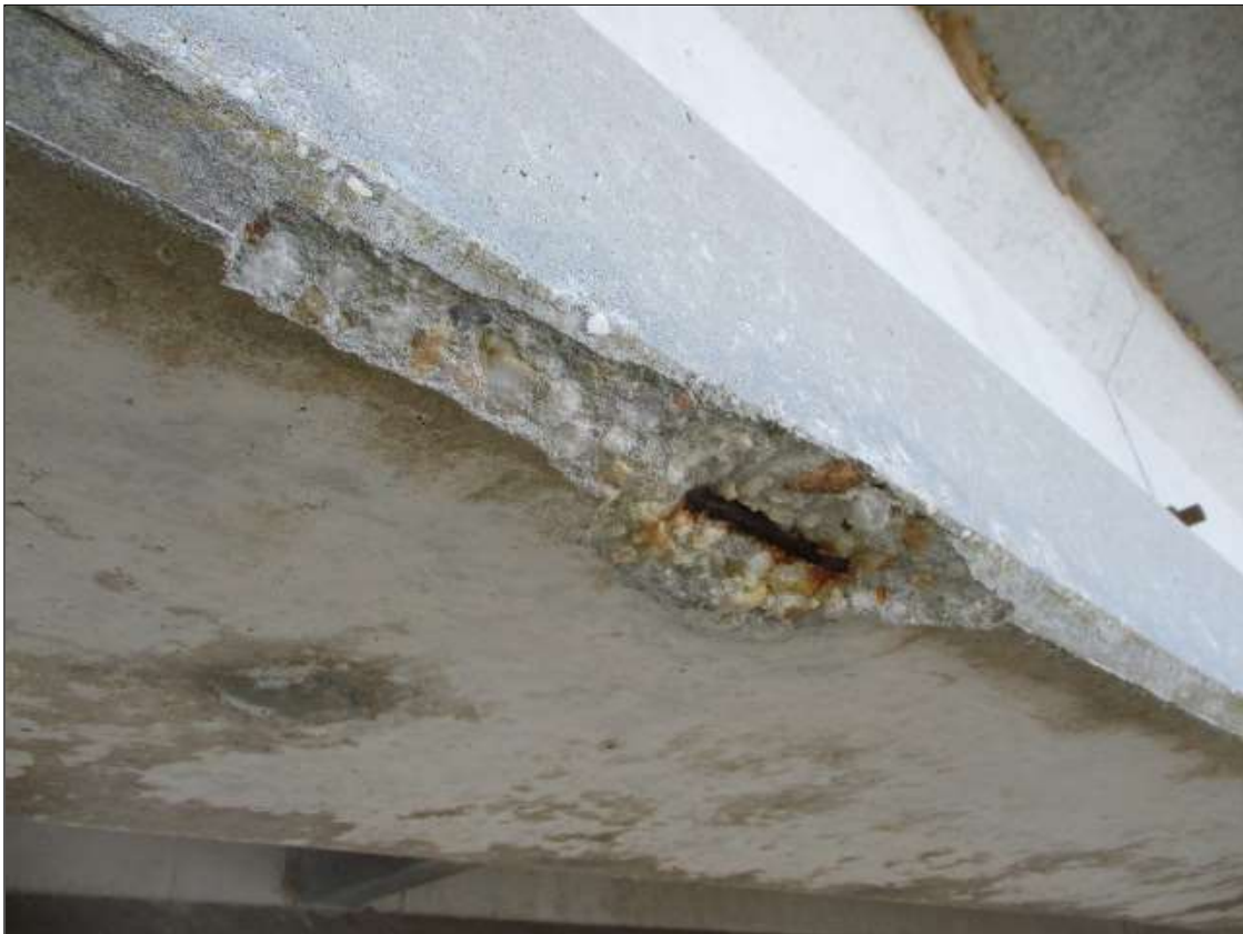
Span 85 Beam 4: SPAN 85 RIGHT BOTTOM EDGE OF BEAM 4. HAS A SPALLED AREA WITH 1 CABLE VISIBLE. LOCATED 24' FROM BENT 85. AREA IS: 5" x 16" x 1" DEEP.
