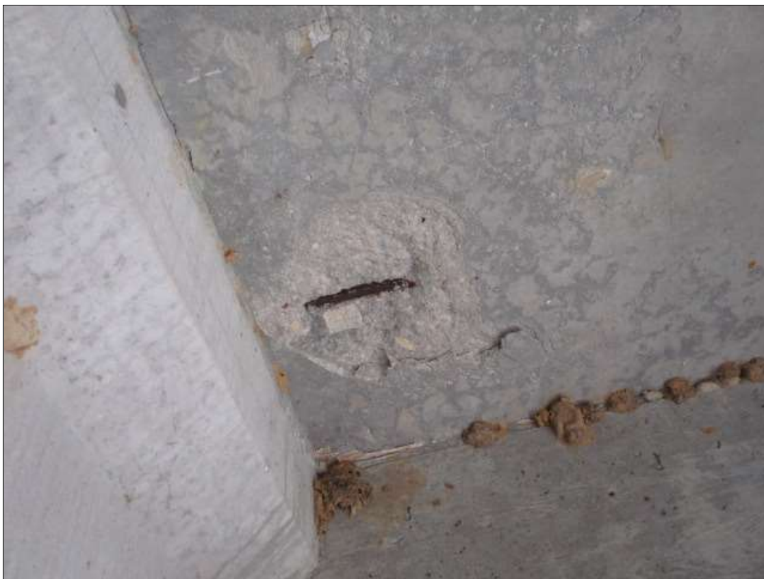
Span 49 Deck: 12" DIAMETER X 1" DEEP SPALL WITH EXPOSED REBAR WITH NO SECTION LOSS IN BAY 3 AT THE 1ST INTERMEDIATE DIAPHRAGM
