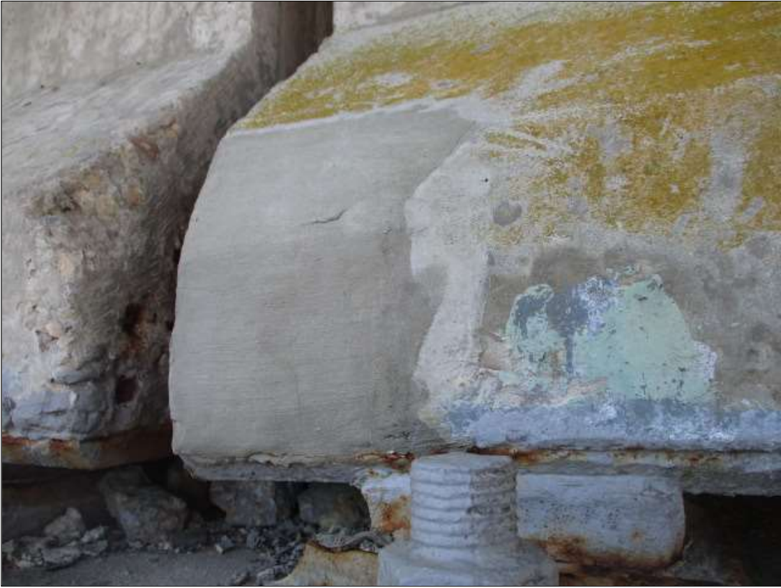
Span 66 Beam 4: SPAN 66 BEAM 4 RIGHT BOTTOM FLANGE OVER BENT 65. sound patch [8in x 8in]
