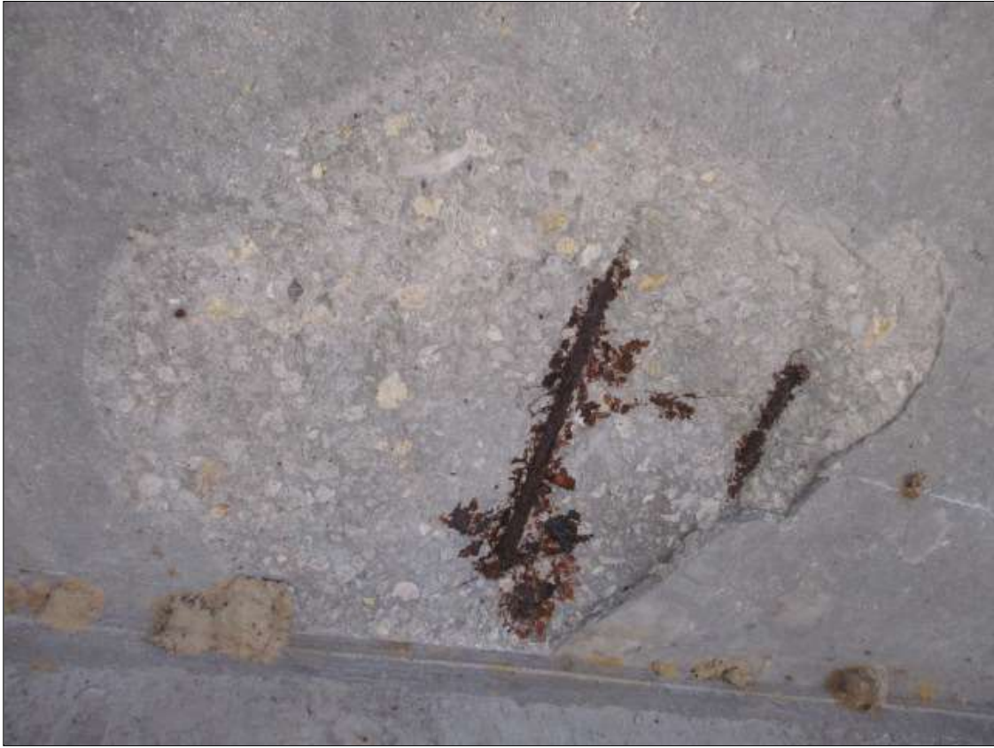
Span 42 Deck: PAR: 30" DIAMETER X 2" DEEP SPALL WITH EXPOSED REBAR WITH SECTION LOSS IN BAY 1 AT 12' FROM BENT 41
