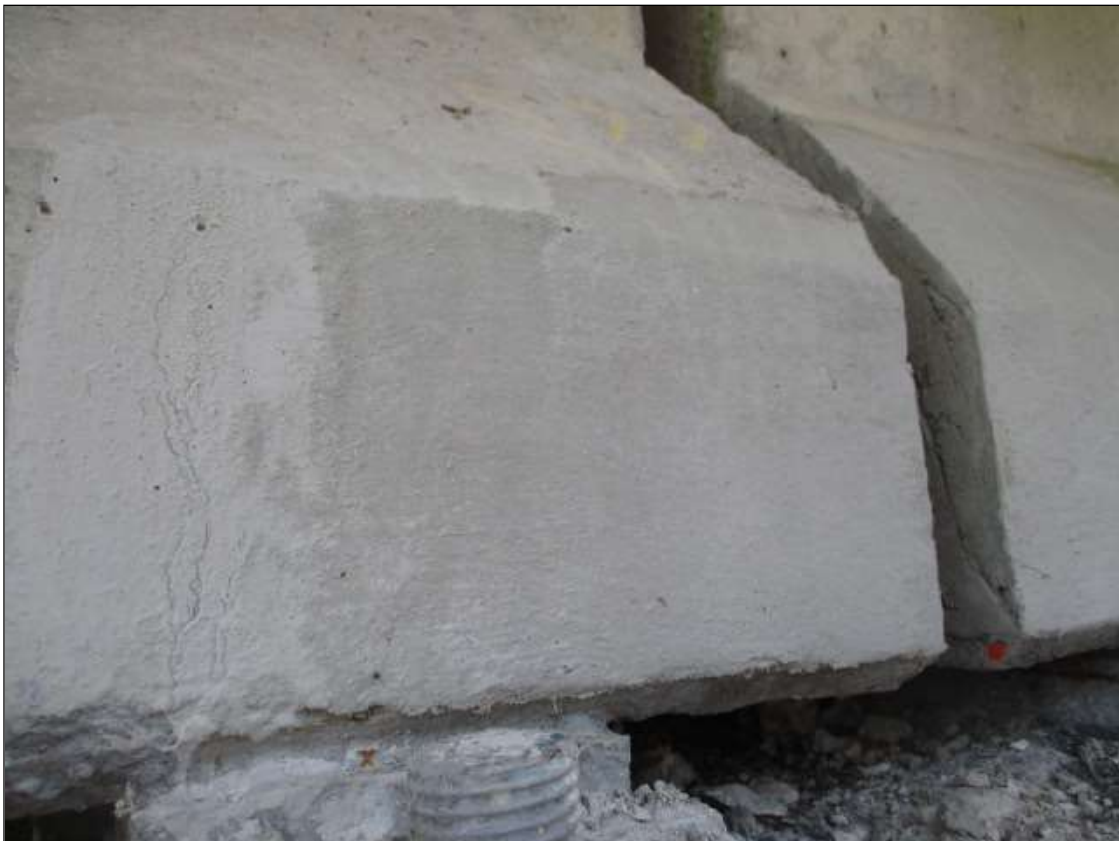
Span 77 Beam 1: 10" LONG X 10" TALL NEW REPAIR TO BOTTOM LEFT FLANGE AT BENT 76
