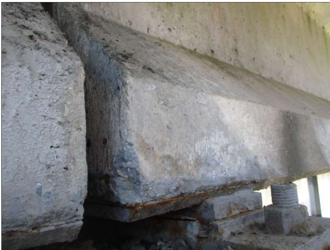
NO SPALL ON BOTTOM LEFT FLANGE OF GIRDER 1 SPAN 77 AT BENT 77 (REPAIR AT BENT 76)
