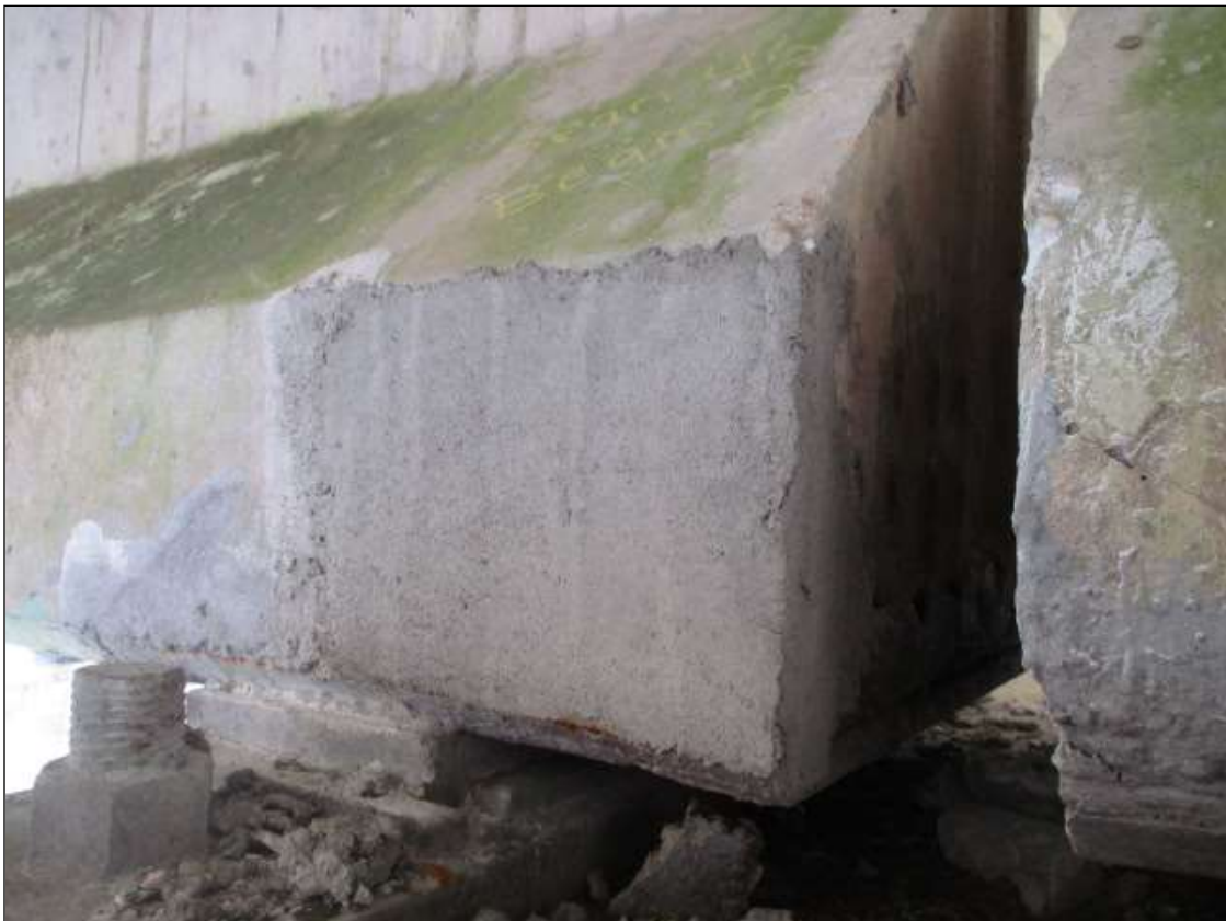
Span 45 Beam 2: 10" LONG X 10" TALL NEW REPAIR TO BOTTOM RIGHT FLANGE AT BENT 45
