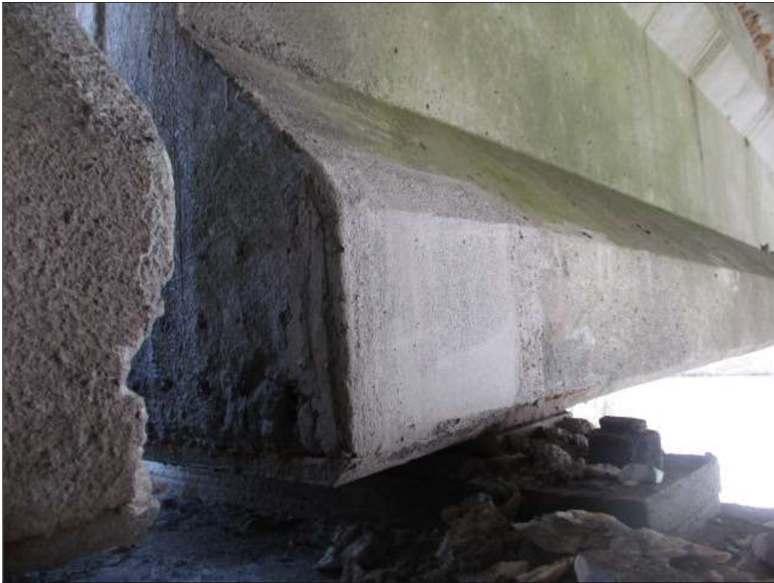
Span 25 Beam 4: 10" LONG X 10" TALL NEW REPAIR TO BOTTOM LEFT FLANGE AT BENT 25
