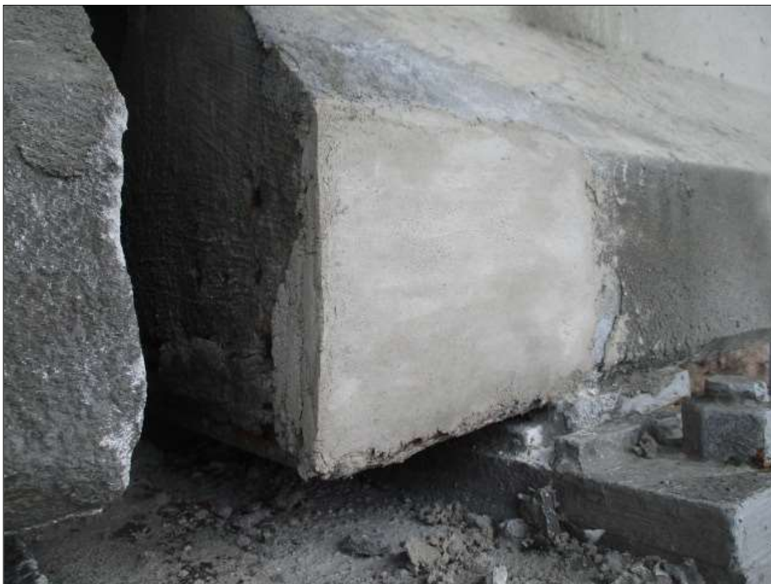
Span 25 Beam 1: 10" LONG X 10" TALL NEW REPAIR TO BOTTOM LEFT FLANGE AT BENT 25
