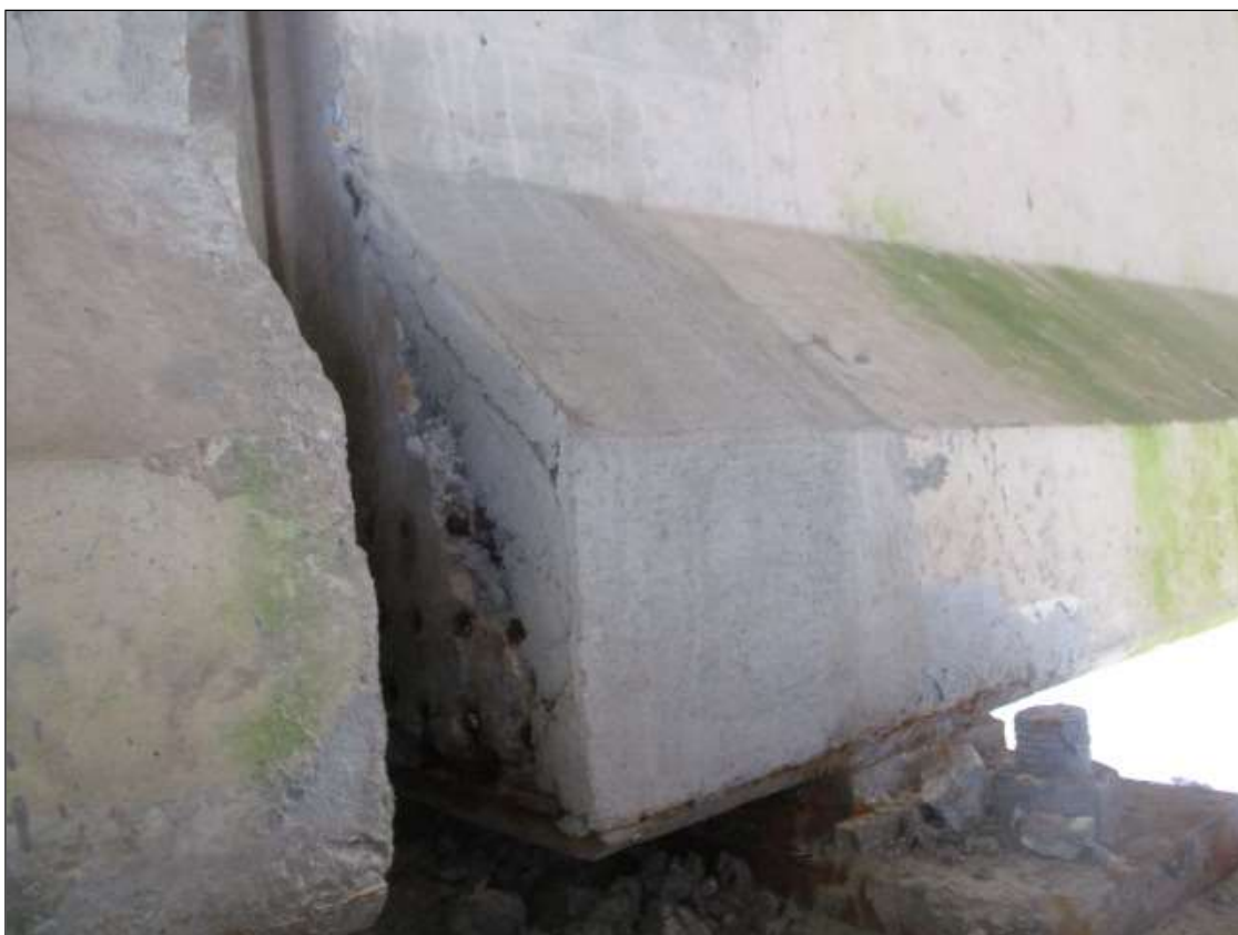
Span 43 Beam 2: 10" LONG X 18" TALL NEW REPAIR TO BOTTOM LEFT FLANGE AT BENT 43
