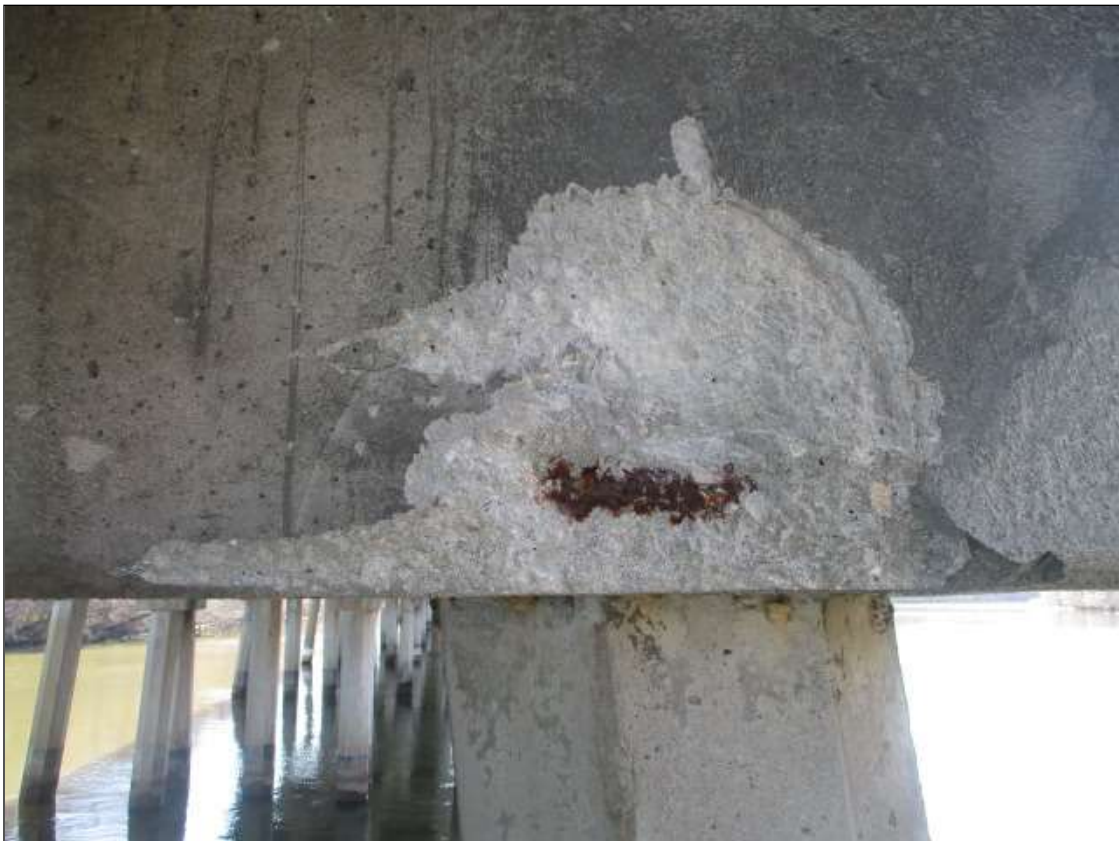
Bent 63 Cap 1: 30" LONG X 18" TALL X 2" DEEP SPALL WITH EXPOSED REBAR WITH NO SECTION LOSS ON NORTH FACE UNDER GIRDER 1
