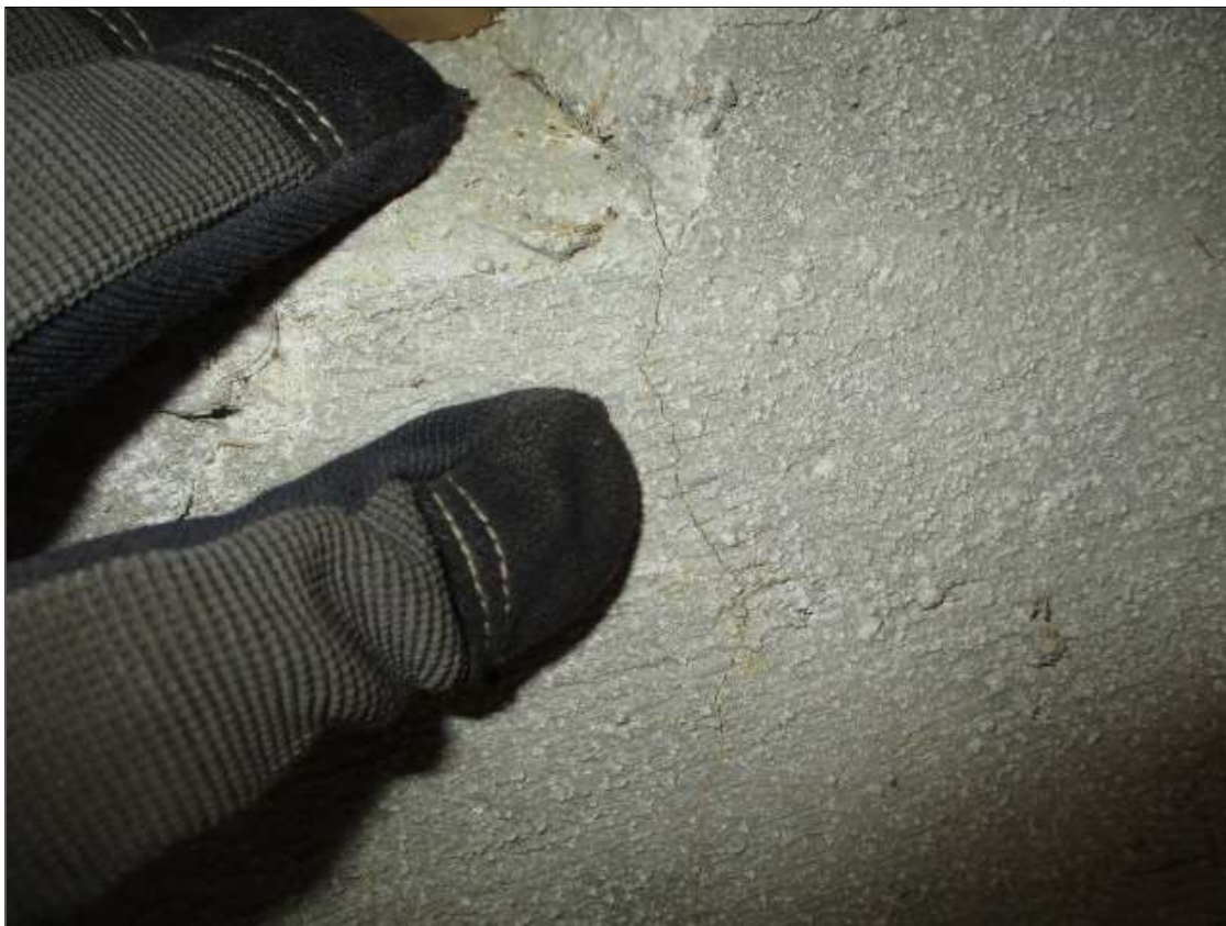
Bent 1 Cap 1: 1/32" VERTICAL CRACKING ON CAP
