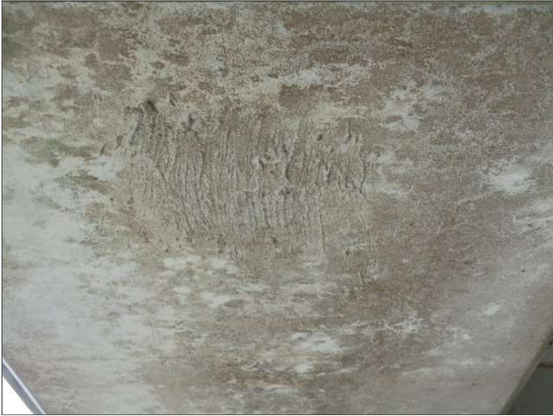
Span 28 Beam 1: 8" LONG X 8" WIDE NEW REPAIR TO UNDERSIDE OF BOTTOM FLANGE AT 8' FROM BENT 27
