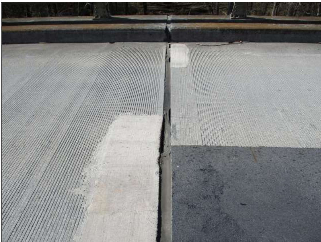
Span 39 Expansion Joint over Bent 38: in left lane, loss of seal adhesion [up to 3ft x full depth]
