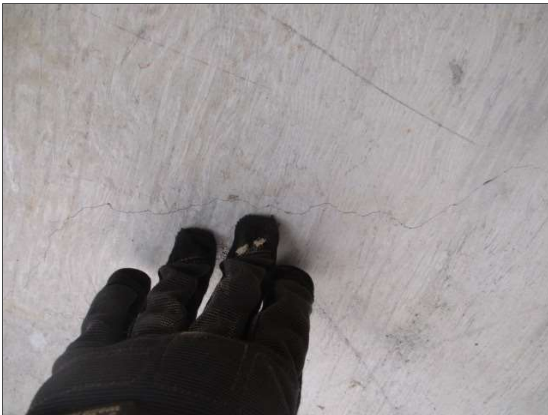
Span 53 Deck: SPAN 53 BOTTOM OF DECK HAS SCATTERED MAP CRACKING.
