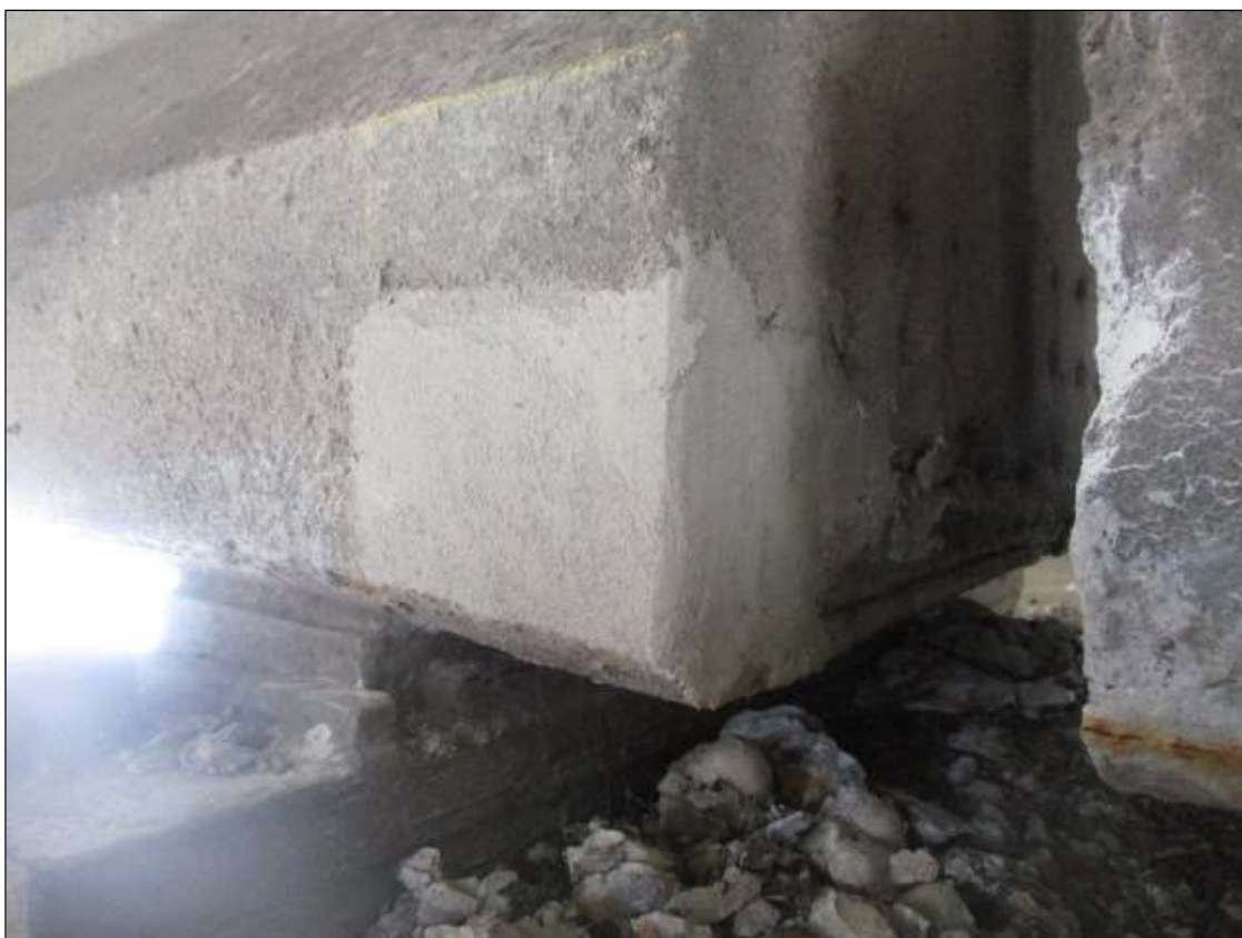
Span 28 Beam 3: 6" LONG X 4" TALL NEW REPAIR TO BOTTOM RIGHT FLANGE AT BENT 28
