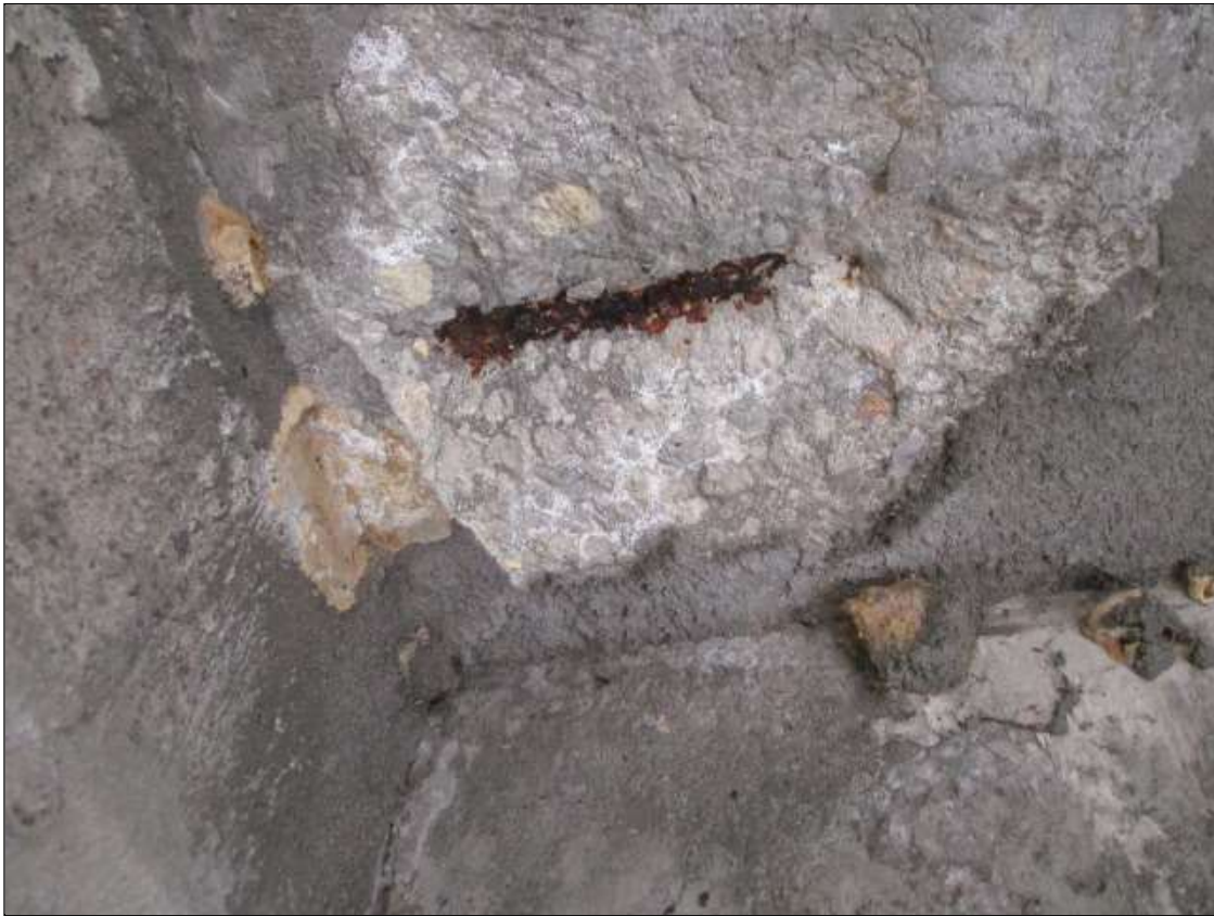
Span 41 Deck: 12" DIAMETER X 1" DEEP SPALL WITH EXPOSED REBAR IN UNDERSIDE OF BAY 1 AT BENT 40
