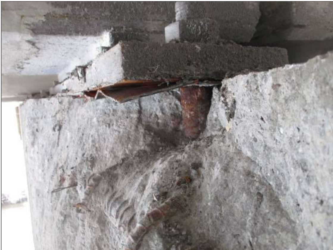
Span 6 Beam 3 Far Bearing: PAR: 18" WIDE X 6" DEEP TRIANGULAR AREA OF LOSS OF BEARING AT BENT 6 CAP DUE TO LARGE SPALL ON SOUTH FACE OF CAP
