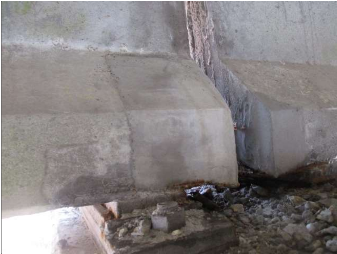
Span 4 Beam 4: 10" LONG X 8" TALL NEW PATCH ON BOTTOM LEFT FLANGE AT BENT 3
