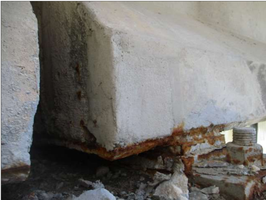
Span 69 Beam 1: 6" LONG X 6" TALL NEW REPAIR TO BOTTOM LEFT FLANGE AT BENT 69
