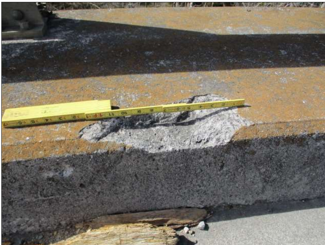
Span 36 Left Bridge Rail: 12" LONG X 6" WIDE X 1" TALL SPALL ON LEFT CURB AT 5' FROM BENT 35
