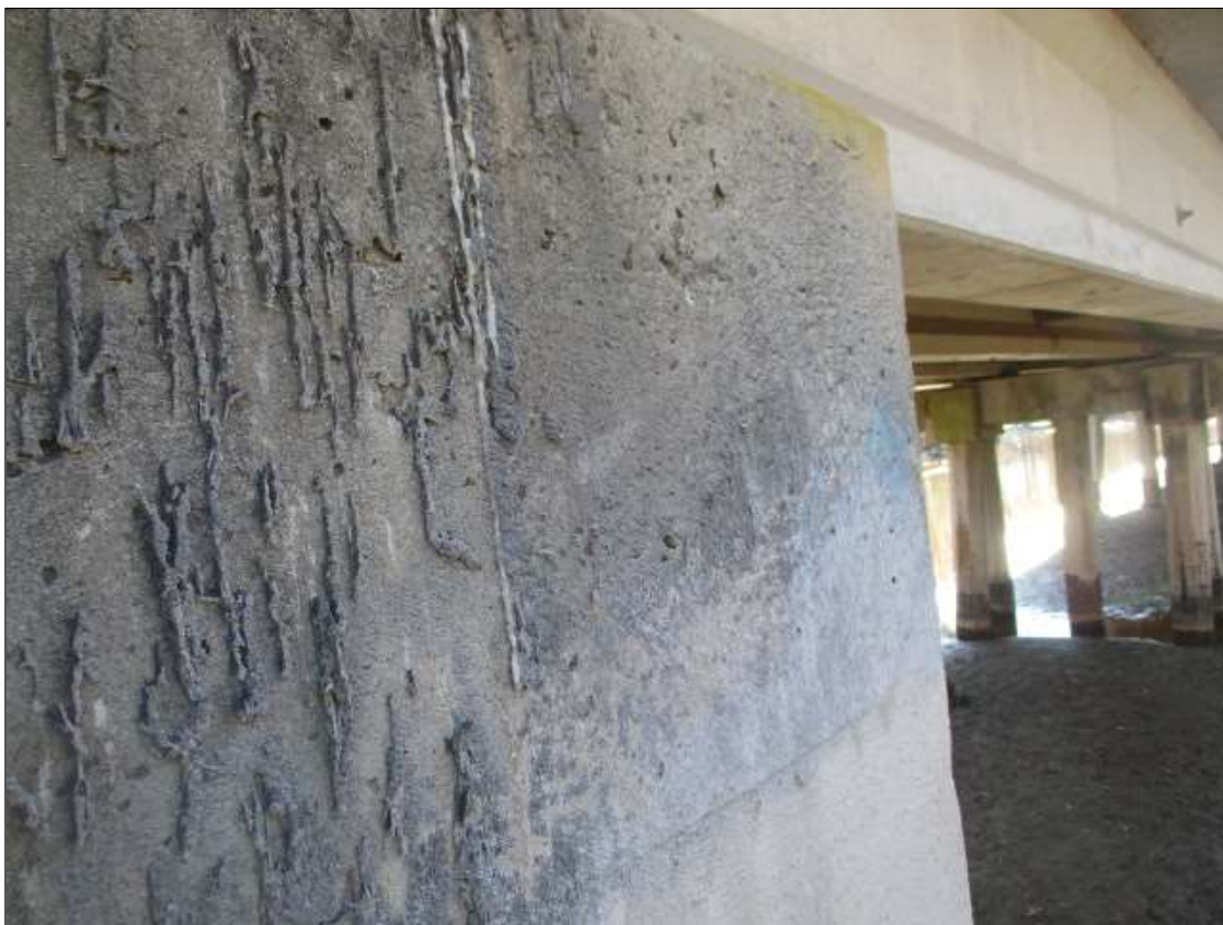
Bent 51 Cap 1: 18" WIDE X 18" TALL NEW REPAIR ON WEST FACE OF CAP
