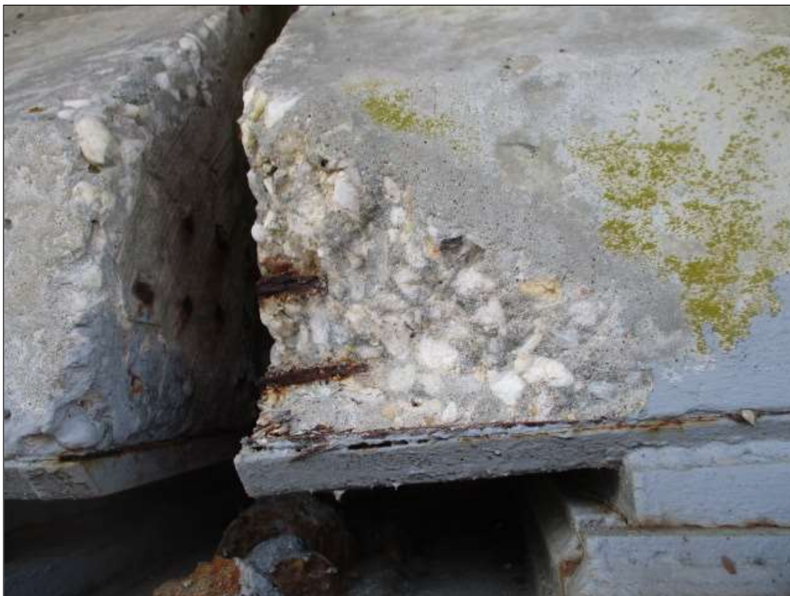
Span 11 Beam 4: East face of bottom flange at bent 10, SPALL [8in x 8in] WITH EXPOSED REBAR WITH NO SECTION LOSS
