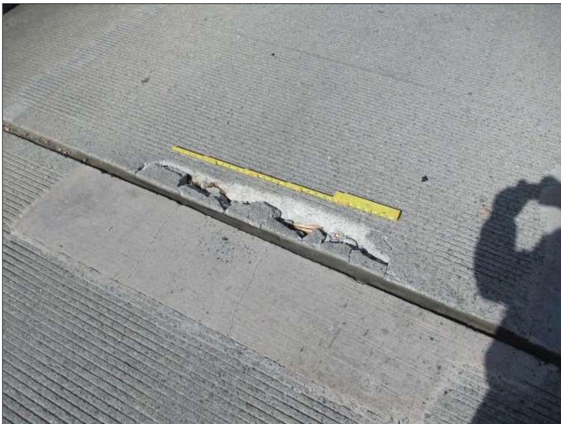
Span 13 Deck: PAR: 3' WIDE X 6" LONG X 3" DEEP SPALL WITH EXPOSED REBAR IN SOUTH BOUND LANE AT BENT 12 JOINT
