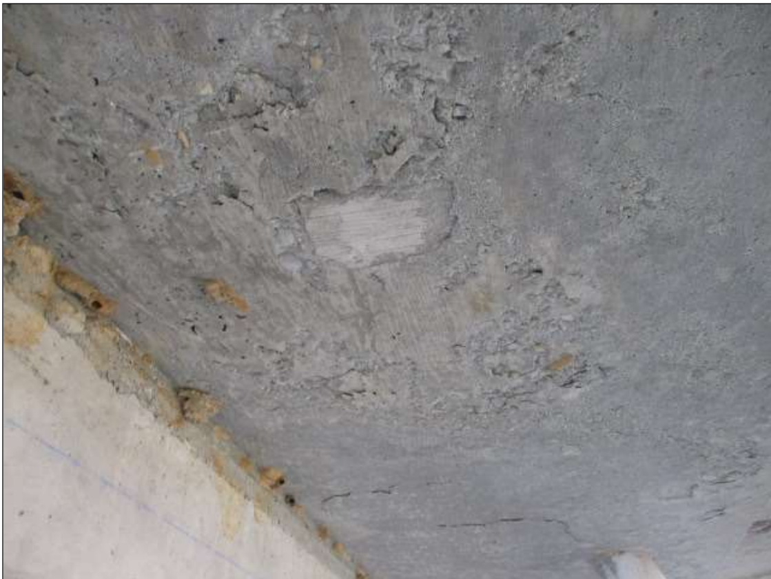
Span 42 Deck: AREA OF POORLY CONSOLIDATED CONCRETE IN RIGHT OVERHANG
