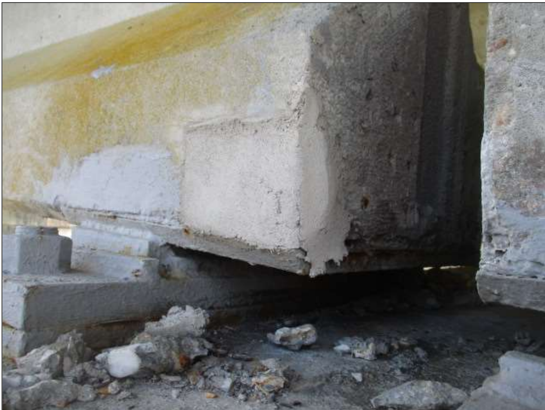
Span 25 Beam 4: 6" LONG X 6" TALL NEW REPAIR TO BOTTOM RIGHT FLANGE AT BENT 25
