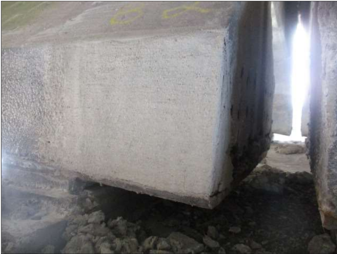
Span 24 Beam 2: 10" LONG X 10" TALL NEW REPAIR TO BOTTOM RIGHT FLANGE AT BENT 24
