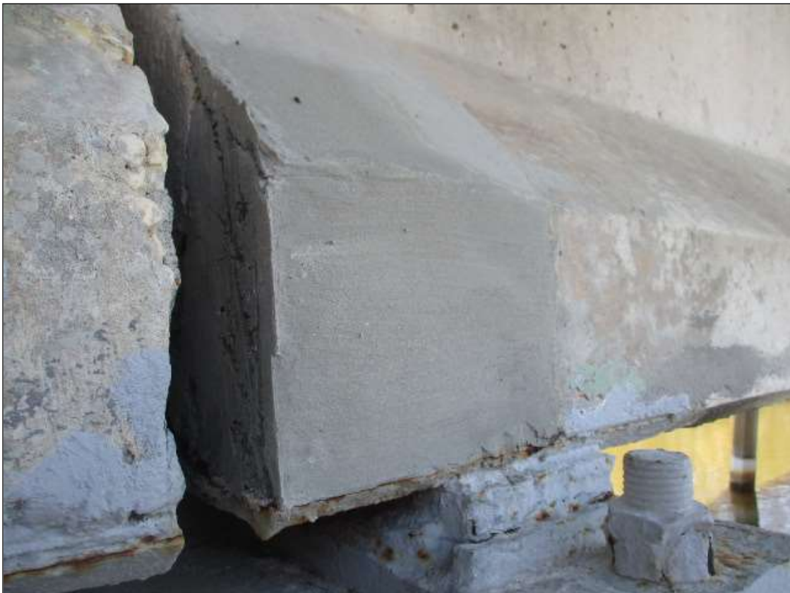
Span 61 Beam 1: SPAN 61 BEAM 1 LEFT BOTTOM FLANGE OVER BENT 61. sound patch [10in x 11in]
