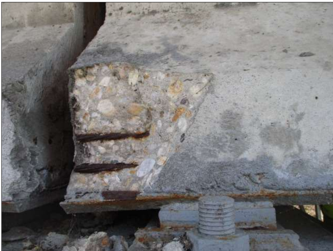
Span 78 Beam 4: bottom right flange at bent 77, spall [8in x 8in x 2in] with [2] two exposed rusted strands [no section loss]
