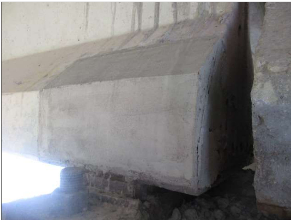
Span 61 Beam 3: 18" LONG X 12" TALL NEW REPAIR TO BOTTOM RIGHT FLANGE AT BENT 61
