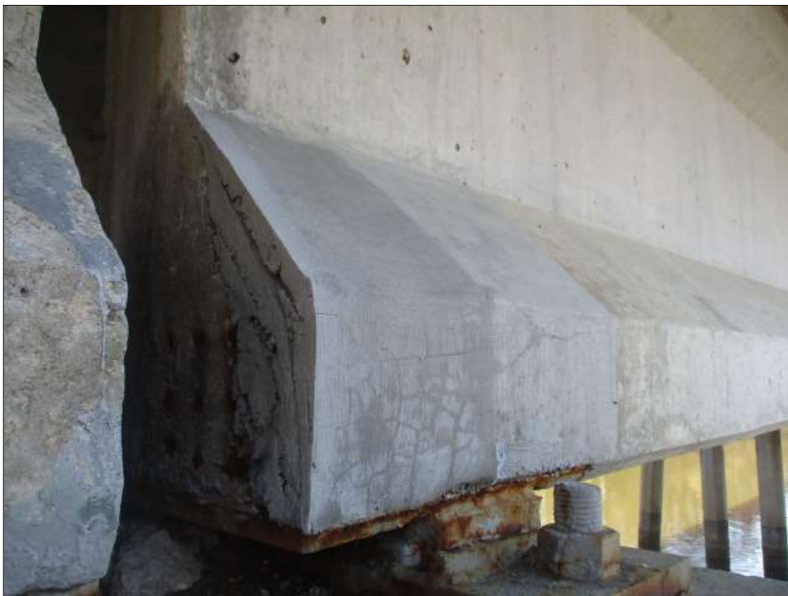
Span 62 Beam 1: SPAN 62 BEAM 1 LEFT BOTTOM FLANGE OVER BENT 62. sound patch [14in x 23in]
