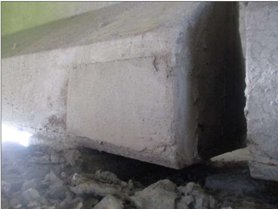
Span 25 Beam 3: 10" LONG X 8" TALL NEW REPAIR TO BOTTOM RIGHT FLANGE AT BENT 25
