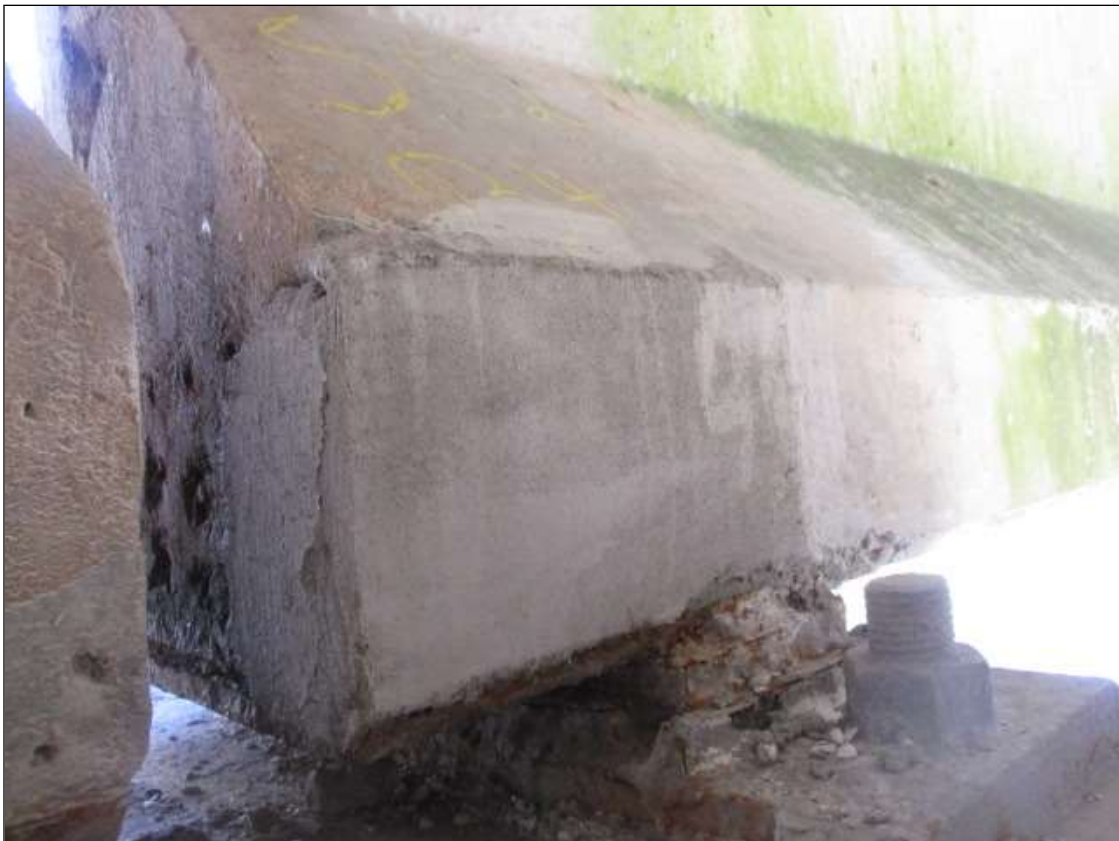
Span 52 Beam 4: 10" LONG X 8" TALL NEW REPAIR TO BOTTOM LEFT FLANGE AT BENT 52
