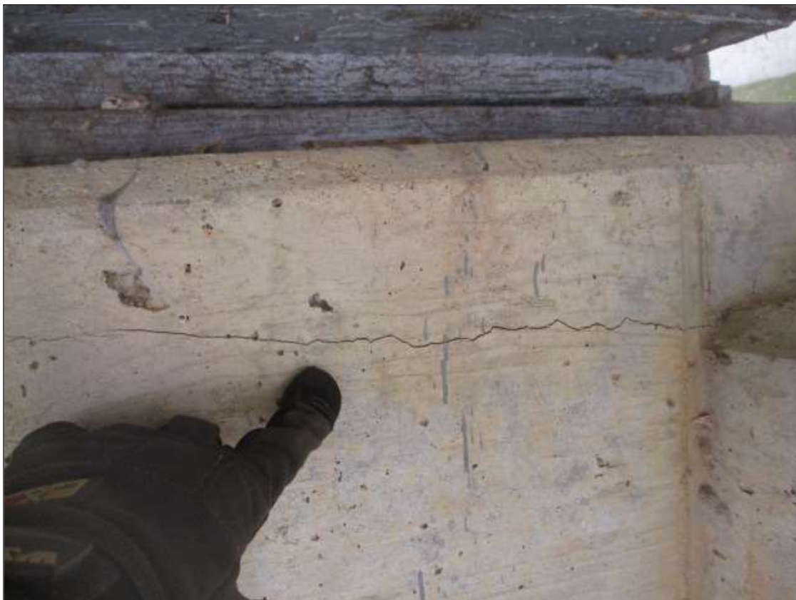
Bent 47 Cap 1: 1/8" HORIZONTAL CRACKING ON NORTH FACE UNDER GIRDER 2
