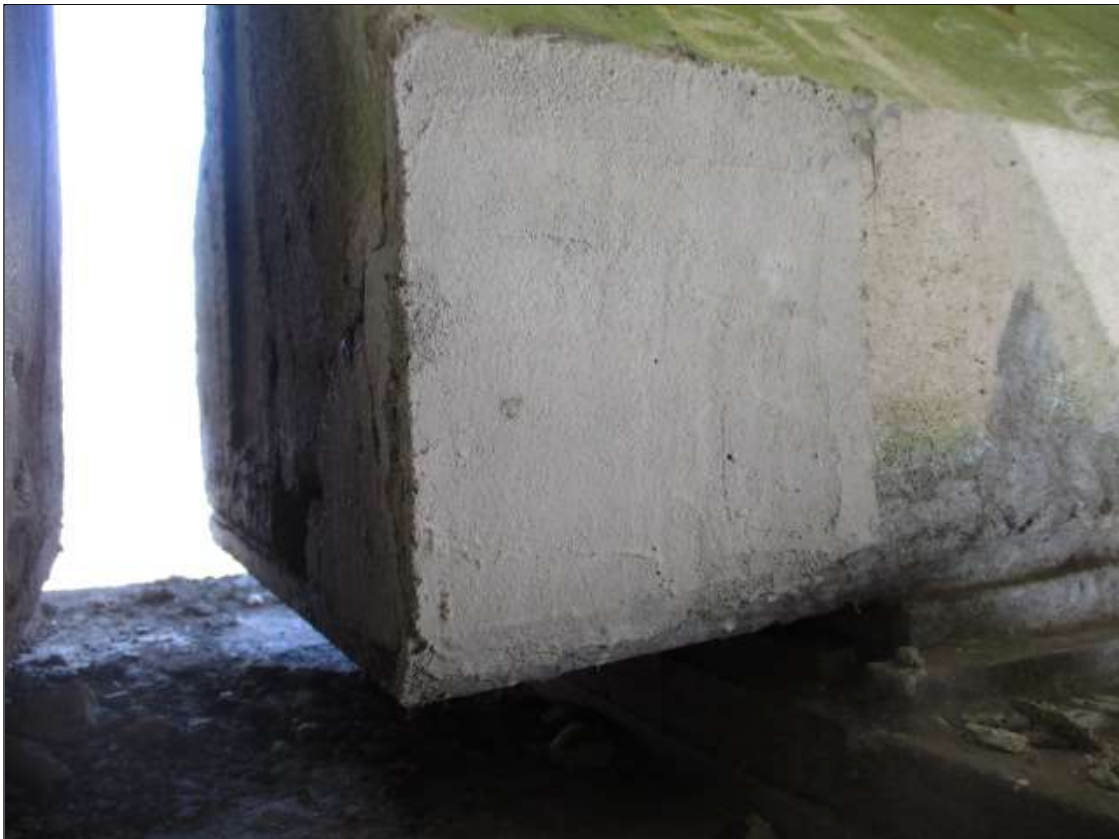
Span 24 Beam 4: 8" LONG X 8" TALL NEW REPAIR TO BOTTOM LEFT FLANGE AT BENT 24
