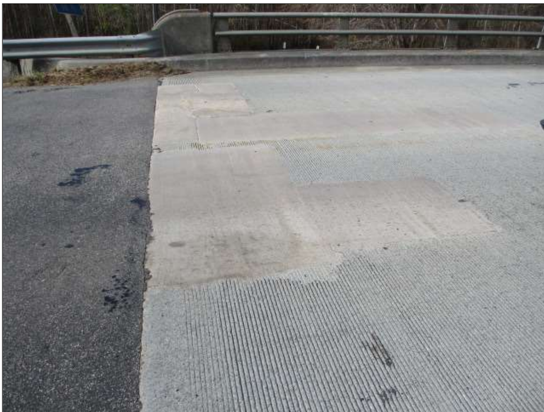
Span 1 Deck: throughout both lanes, multiple sound patches [up to 6ft x up to 8ft]
