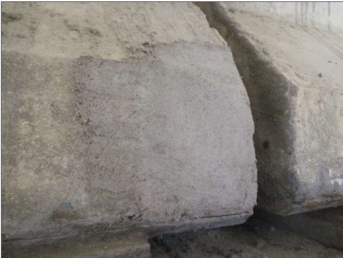
Span 53 Beam 2: SPAN 53 BEAM 2 LEFT BOTTOM FLANGE OVER BENT 52. sound patch [8in x 10in]
