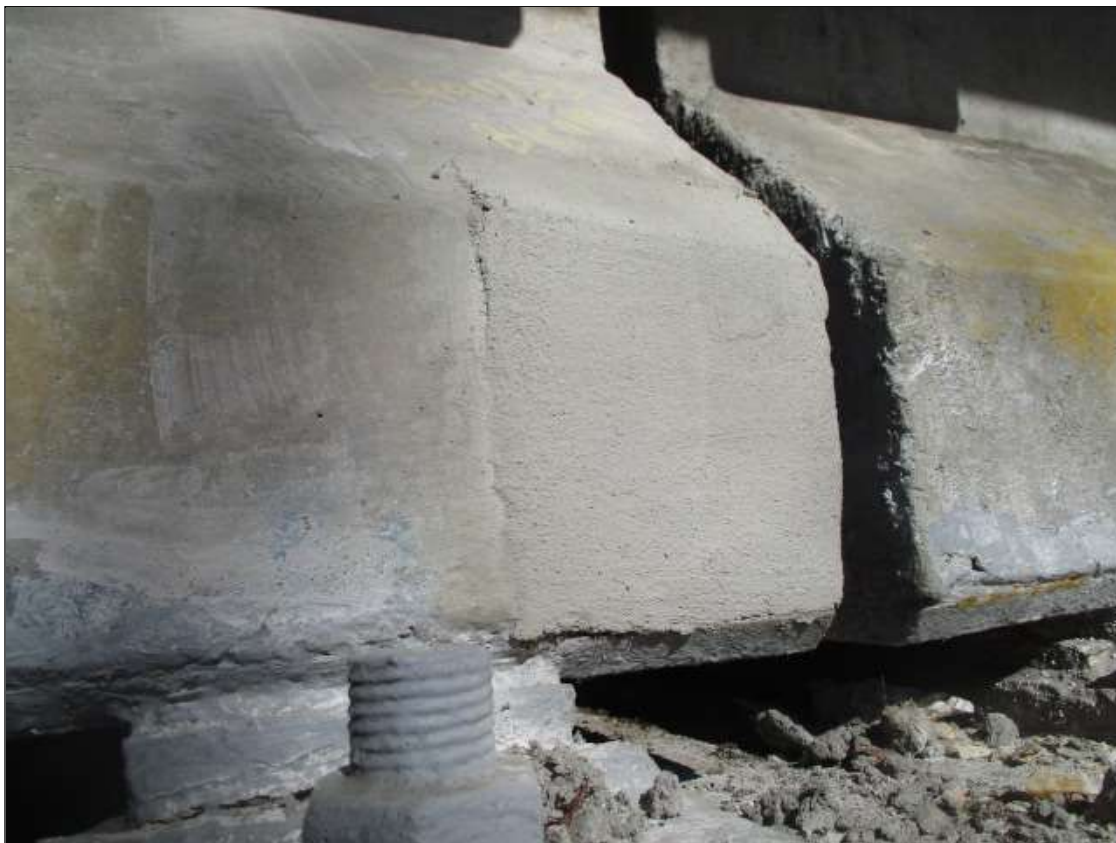
Span 53 Beam 1: 8" LONG X 10" TALL NEW REPAIR TO BOTTOM LEFT FLANGE AT BENT 52
