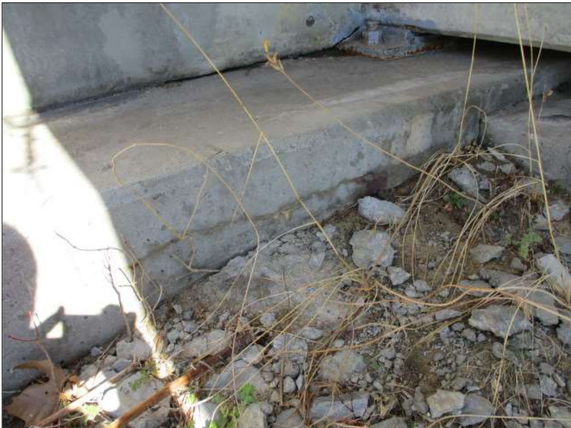
End Bent 2 End Bent 2 Cap: 1/16" HORIZONTAL CRACKING UNDER LEFT OVERHANG
