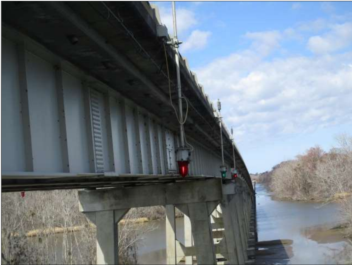
NAVIGATION LIGHTS ON BOTH SIDES OF SPAN 18
