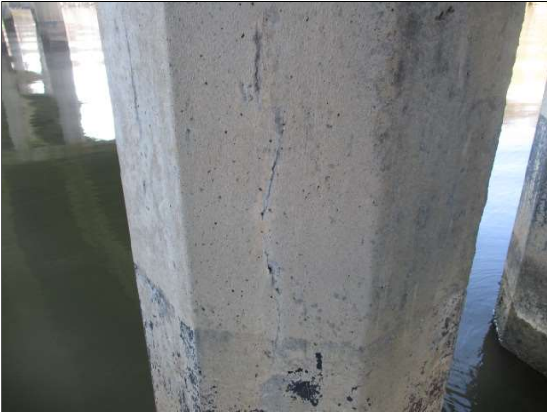
Bent 63 Pile 4: 1/64" VERTICAL CRACKING ON ALL FACES
