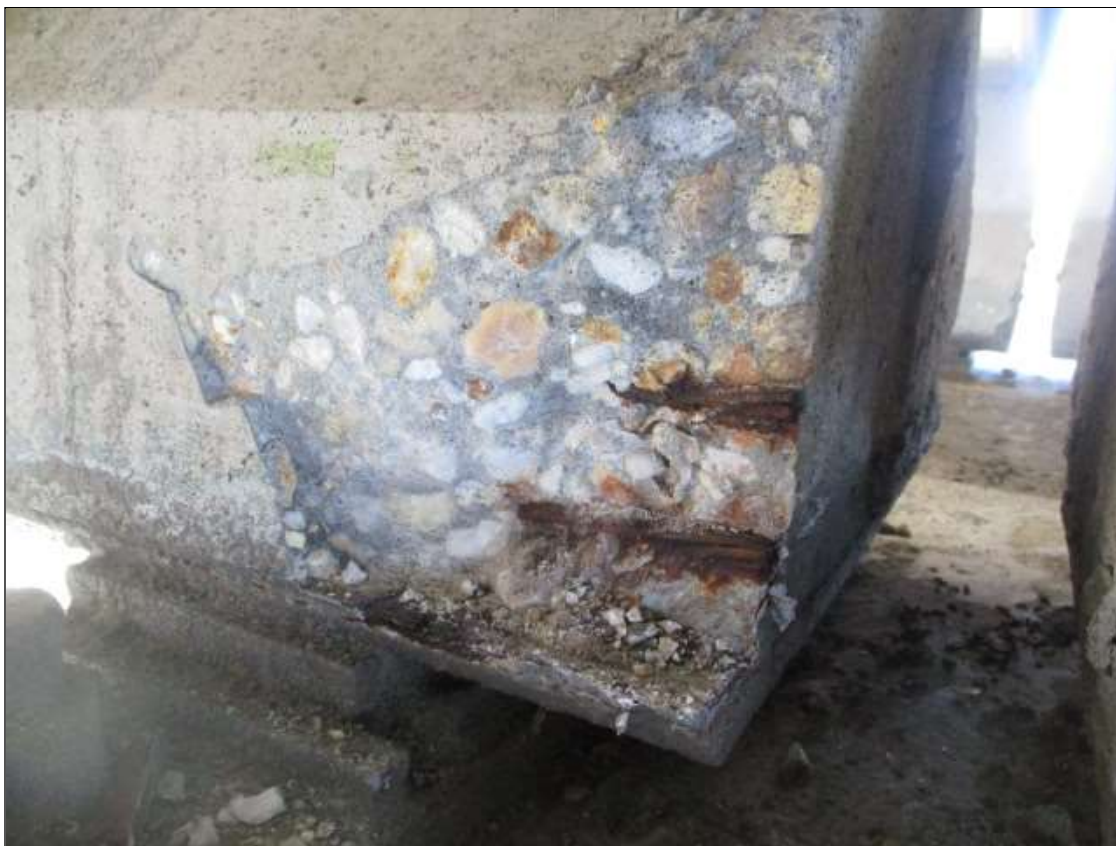
Span 80 Beam 2: SPAN 80 BEAM 2 RIGHT BOTTOM FLANGE OVER BENT 80. HAS A SPALL. AREA IS: 7" x 9" x 2" DEEP.
