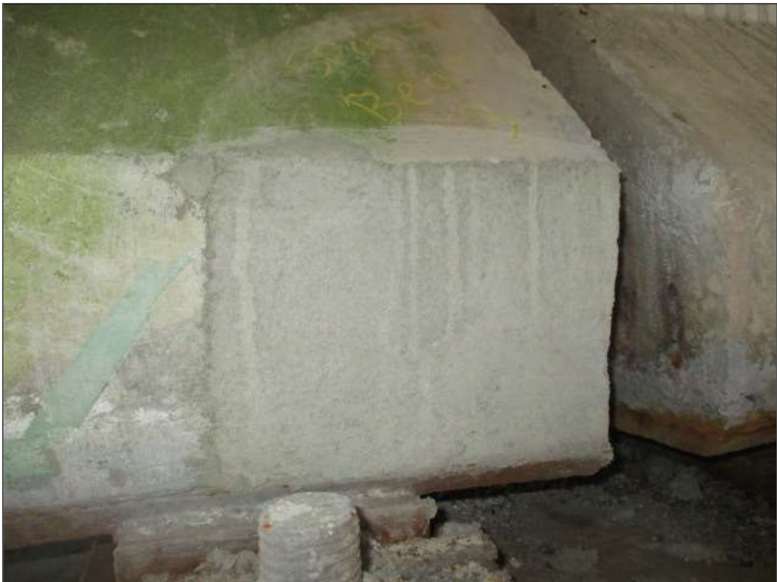
Span 46 Beam 3: 10" LONG X 10" TALL NEW REPAIR TO BOTTOM LEFT FLANGE AT BENT 45
