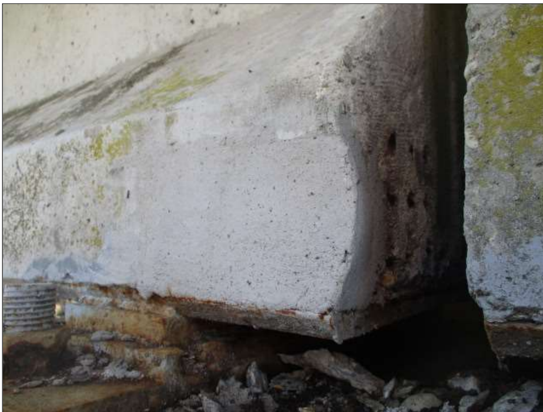
Span 75 Beam 4: 8" LONG X 6" TALL NEW REPAIR TO BOTTOM RIGHT FLANGE AT BENT 75
