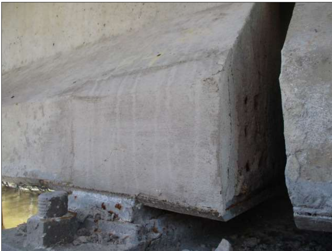
Span 76 Beam 4: 12" LONG X 10" TALL NEW REPAIR TO BOTTOM RIGHT FLANGE AT BENT 76
