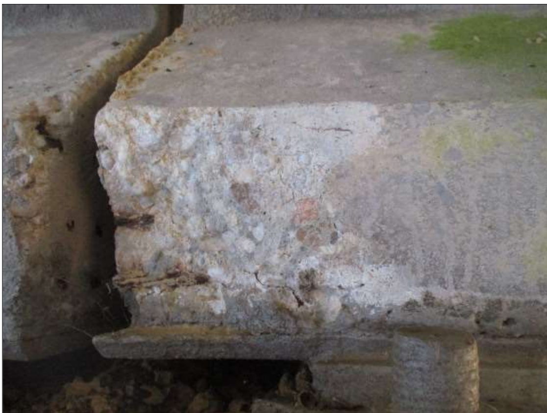
Span 95 Beam 2: 10" LONG X 10" TALL X 2" DEEP SPALL WITH 2 EXPOSED STRANDS WITH NO SECTION LOSS ON BOTTOM RIGHT FLANGE AT BENT 94
