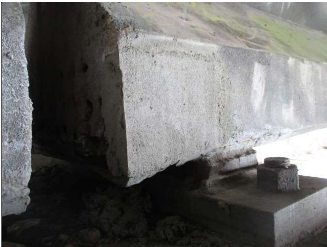
Span 28 Beam 3: 8" LONG X 8" TALL NEW REPAIR TO BOTTOM LEFT FLANGE AT BENT 28
