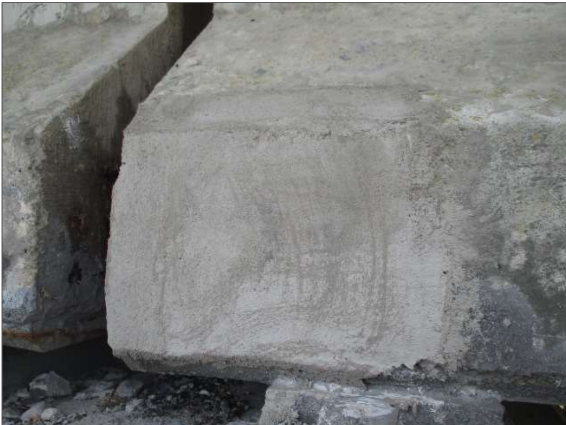
Span 33 Beam 4: 10" LONG X 10" TALL NEW REPAIR TO BOTTOM RIGHT FLANGE AT BENT 32
