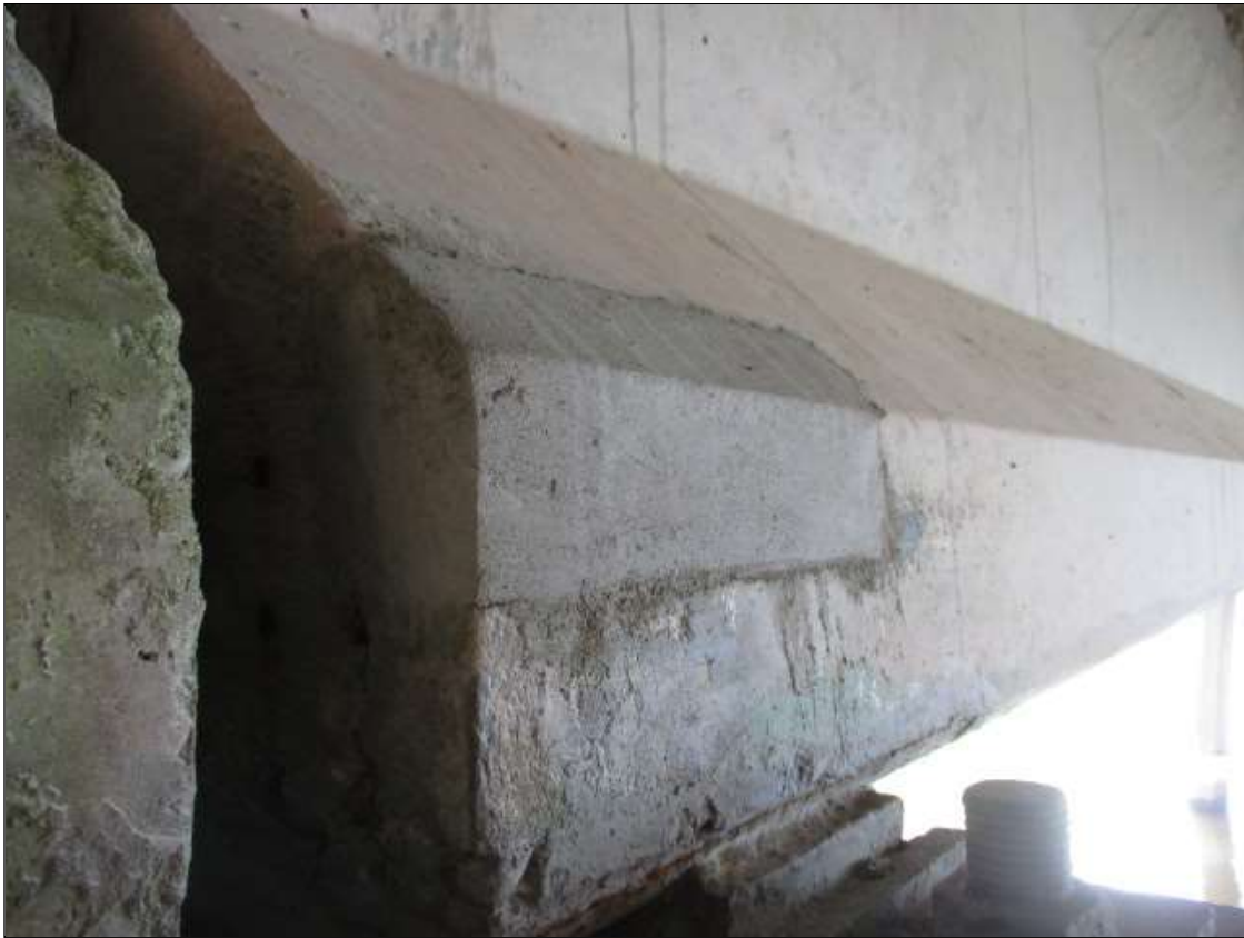
Span 61 Beam 3: 10" LONG X 4" TALL NEW REPAIR TO BOTTOM LEFT FLANGE AT BENT 61
