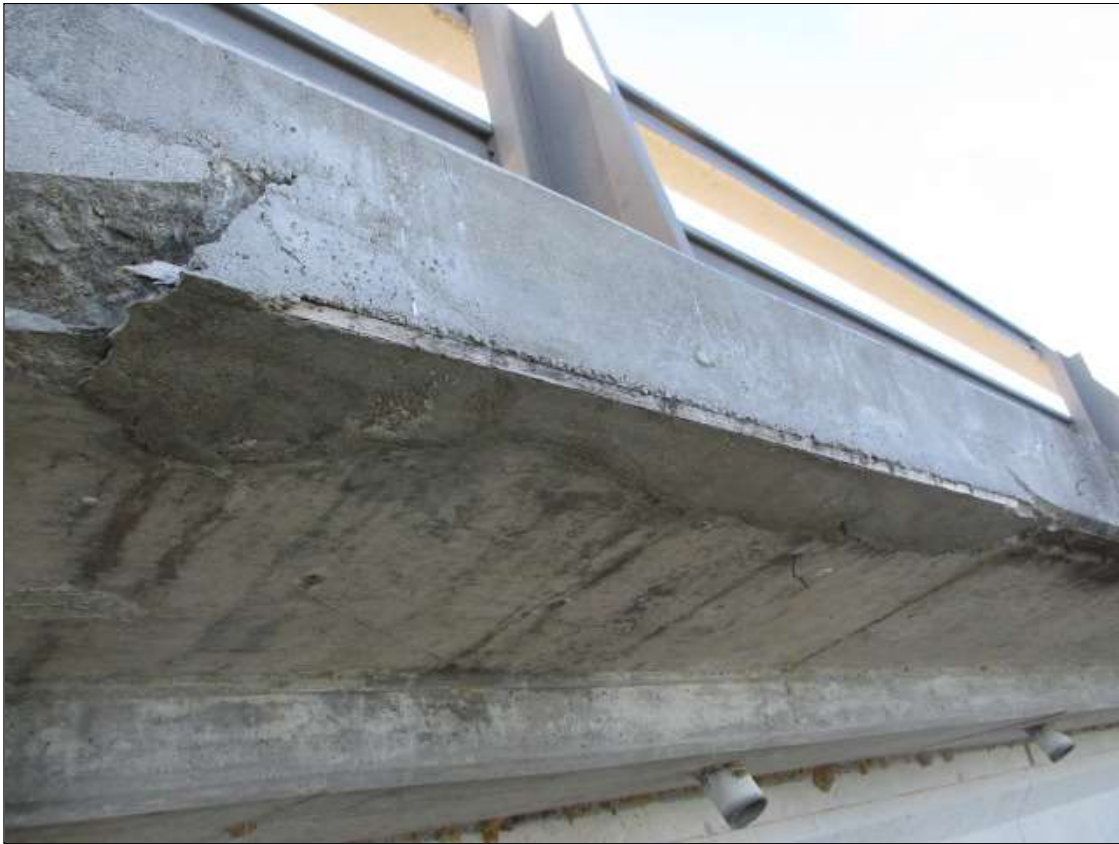
Span 85 Deck: 4' LONG X 8" TALL X 8" WIDE DELAMINATED PATCH IN RIGHT OVERHANG 15' FROM BENT 84
