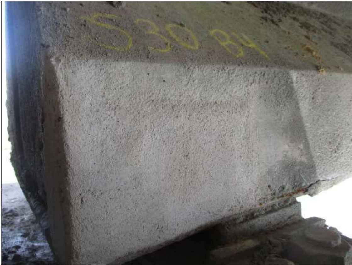
Span 30 Beam 4: 8" LONG X 8" TALL NEW REPAIR TO BOTTOM LEFT FLANGE AT BENT 30
