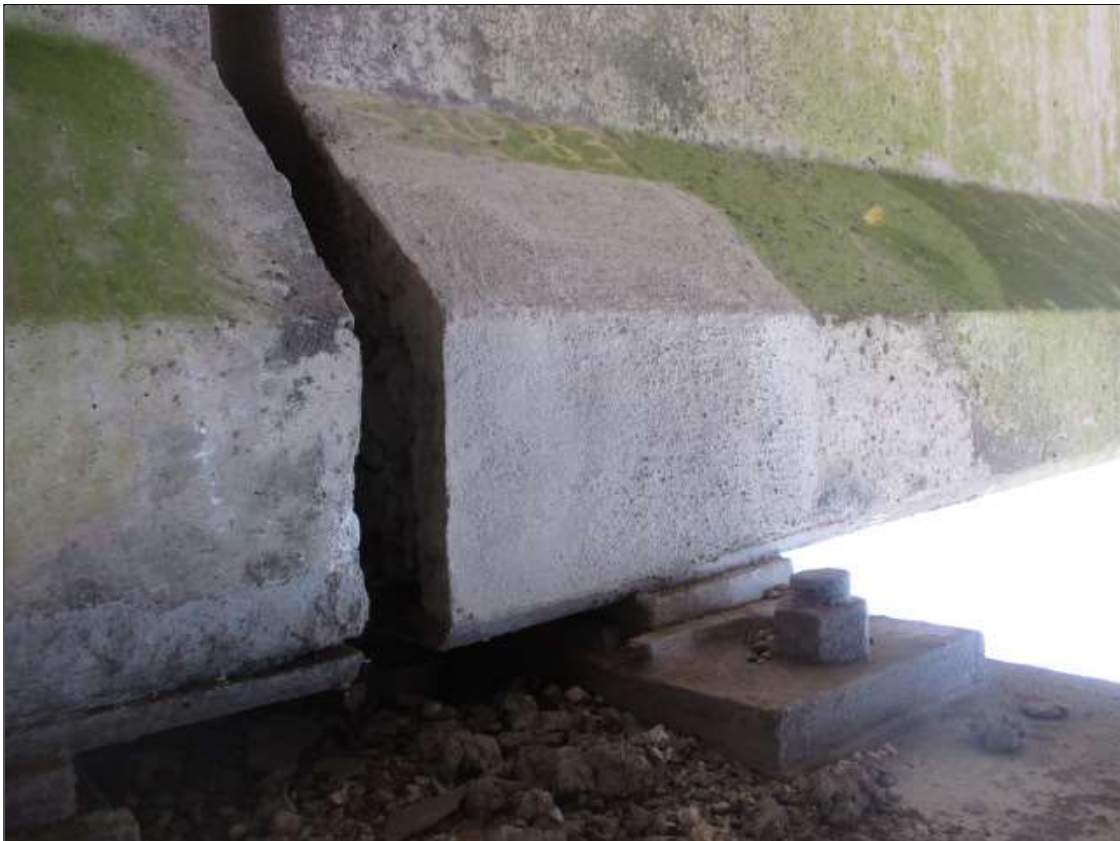
Span 21 Beam 3: 8" LONG X 18" TALL NEW REPAIR TO BOTTOM LEFT FLANGE AT BENT 21
