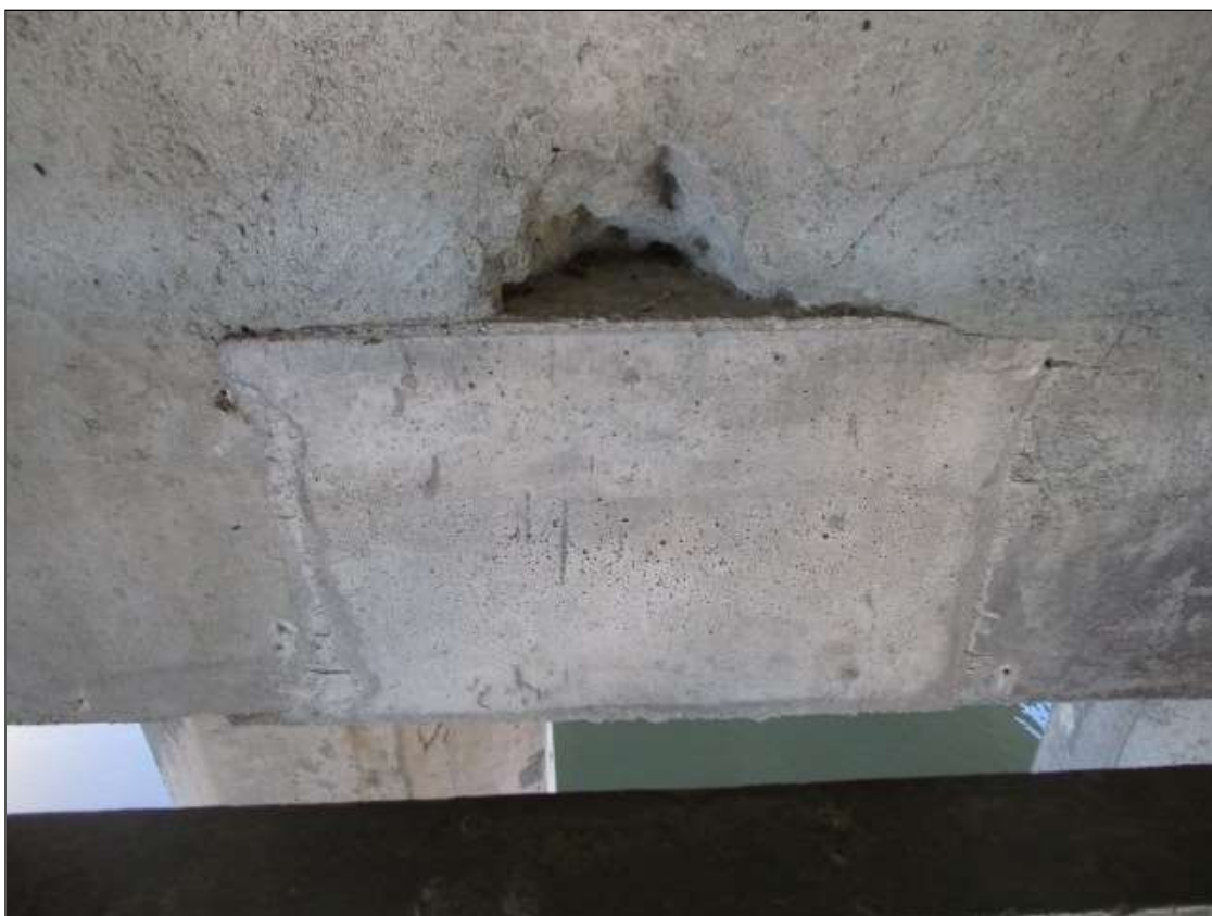
Bent 63 Cap 1: BENT 63 CAP NORTH FACE BAY 2. HAS A SPALLED AREA. AREA IS: 5" x 10" x 4" DEEP.
