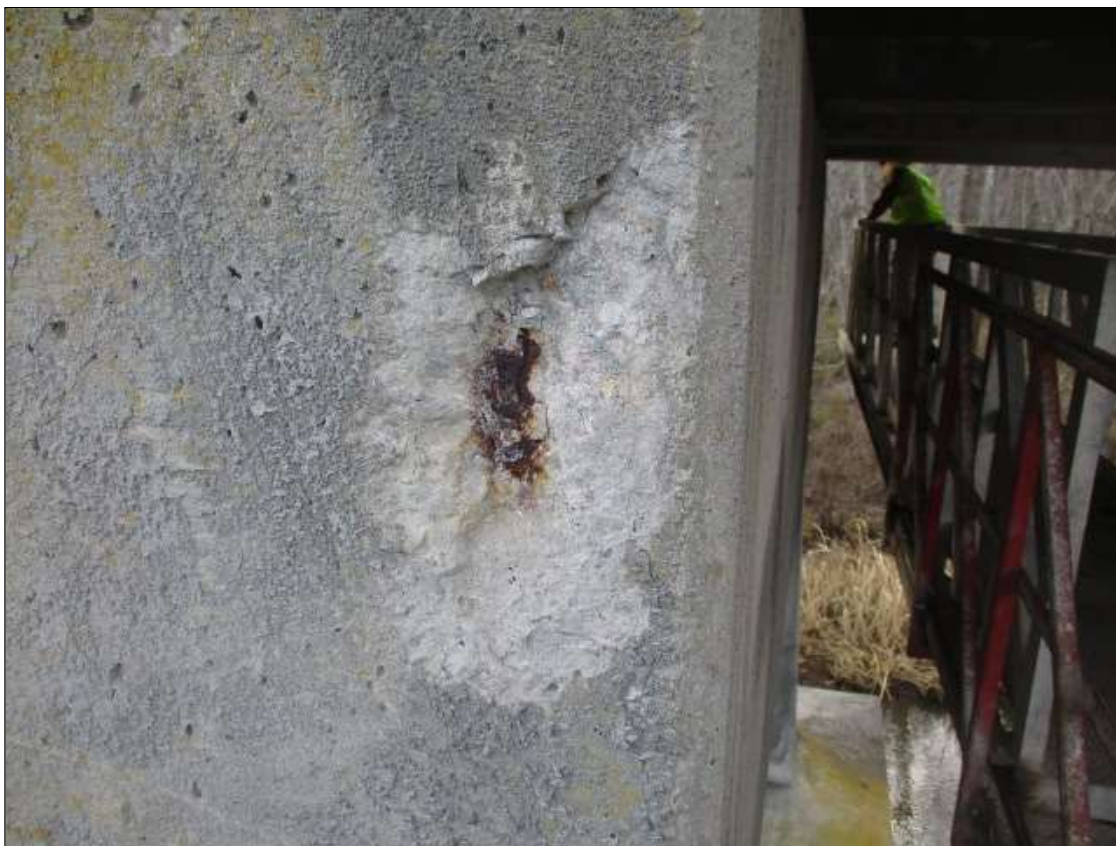
Bent 33 Cap 1: at East end of cap, spall [5in x 9in x up to 1in deep] with [1] one exposed rusted reinforcing [no section loss]
