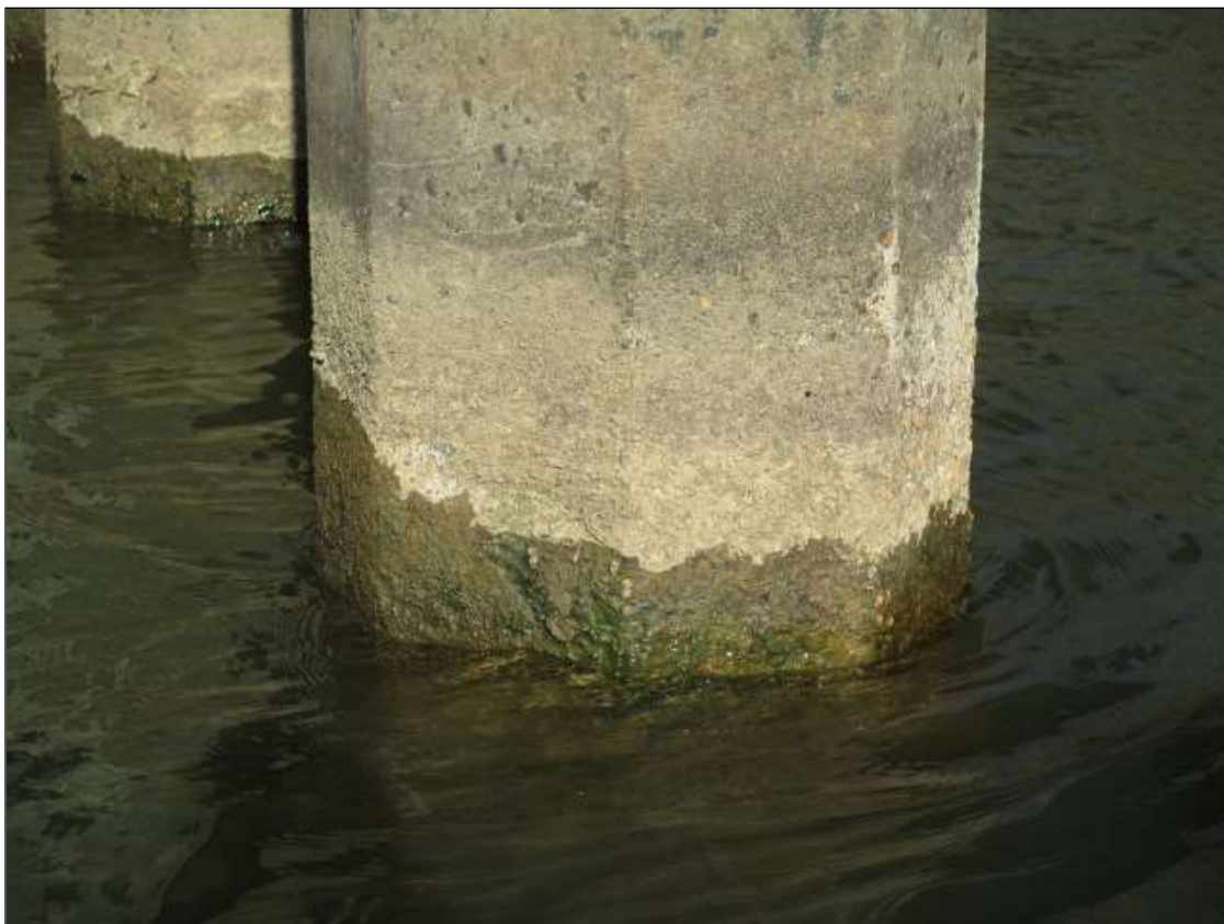
Bent 59 Pile 1: U/W INSPECTION, SCALING 1/2-1" DEEP WITH LOOSE AGGREGATE X 360° FROM WATERLINE DOWN 4'.
