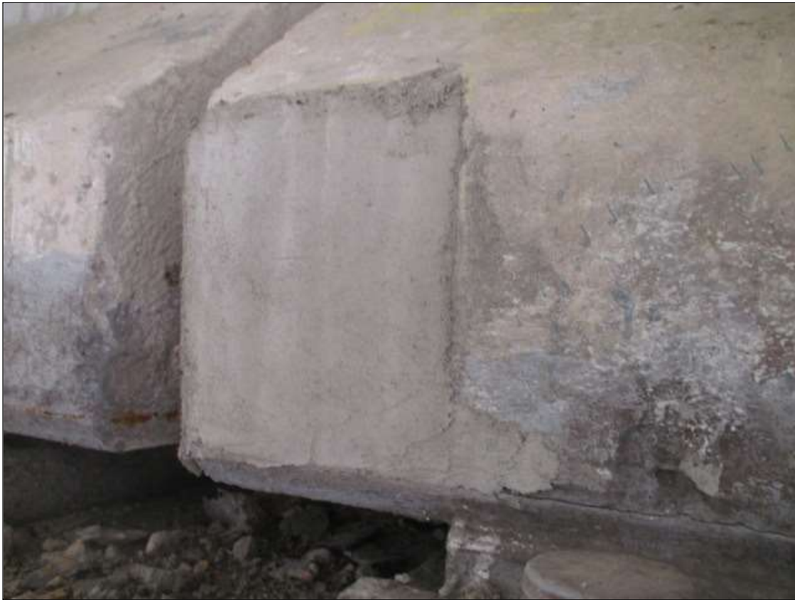
Span 53 Beam 2: 6" LONG X 8" TALL NEW REPAIR TO BOTTOM RIGHT FLANGE AT BENT 52
