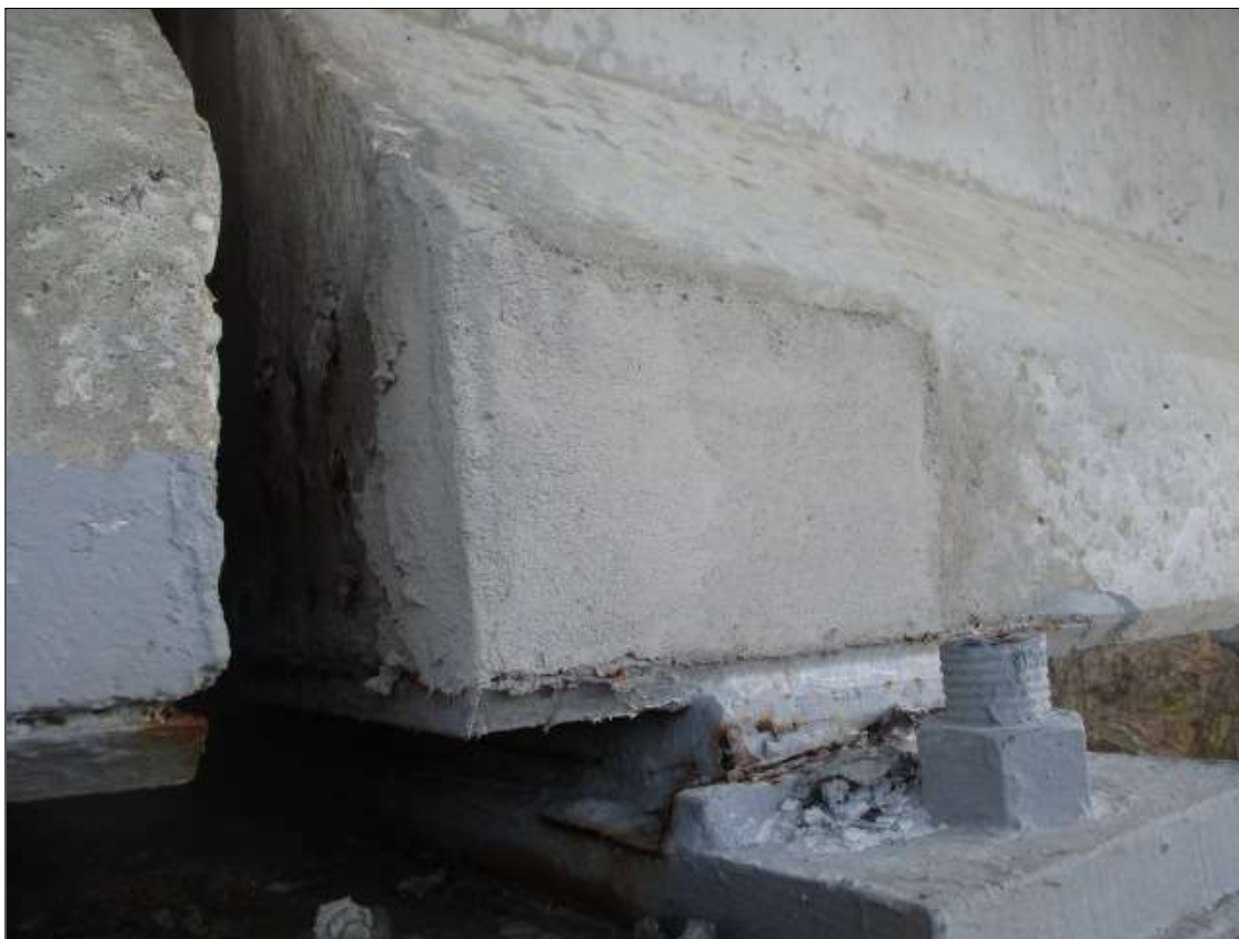
Span 10 Beam 1: 10" LONG X 8" TALL NEW PATCH ON BOTTOM LEFT FLANGE AT BENT 10
