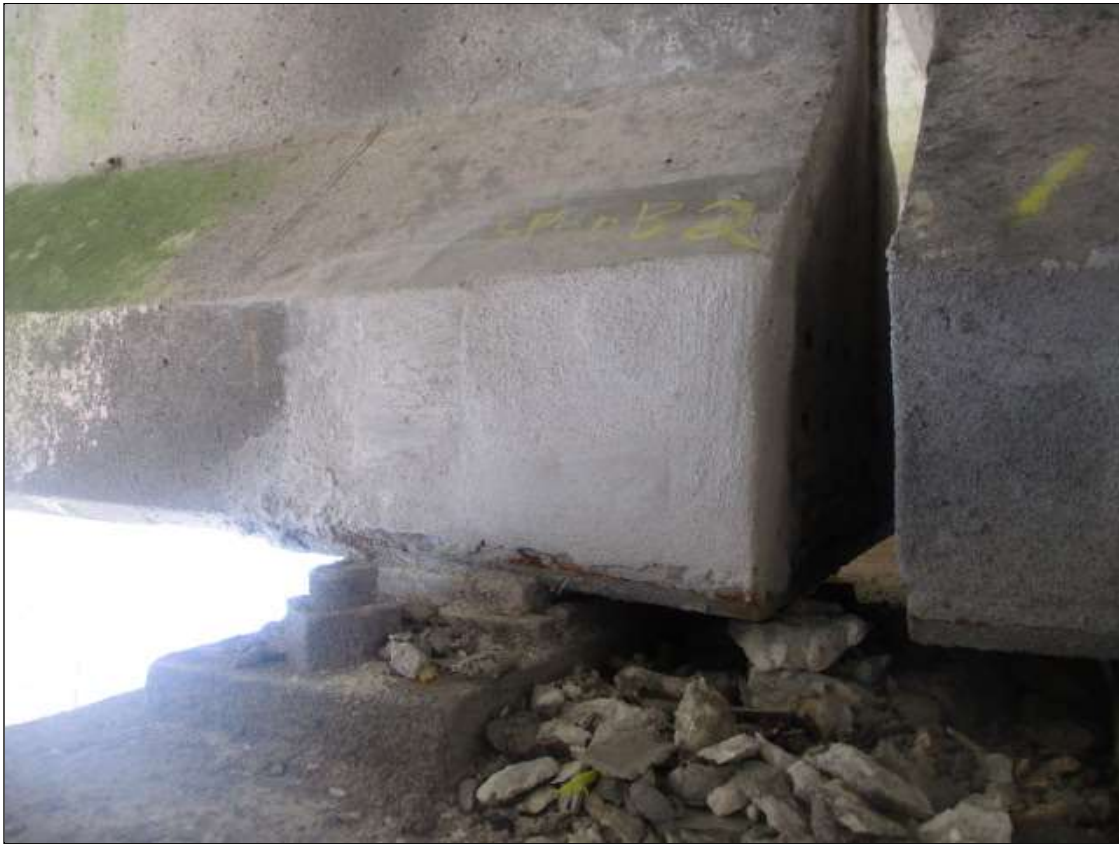
Span 21 Beam 2: 8" LONG X 18" TALL NEW REPAIR TO BOTTOM RIGHT FLANGE AT BENT 21
