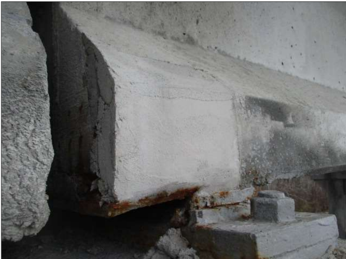
Span 28 Beam 1: 10" LONG X 10" TALL NEW REPAIR TO BOTTOM LEFT FLANGE AT BENT 28
