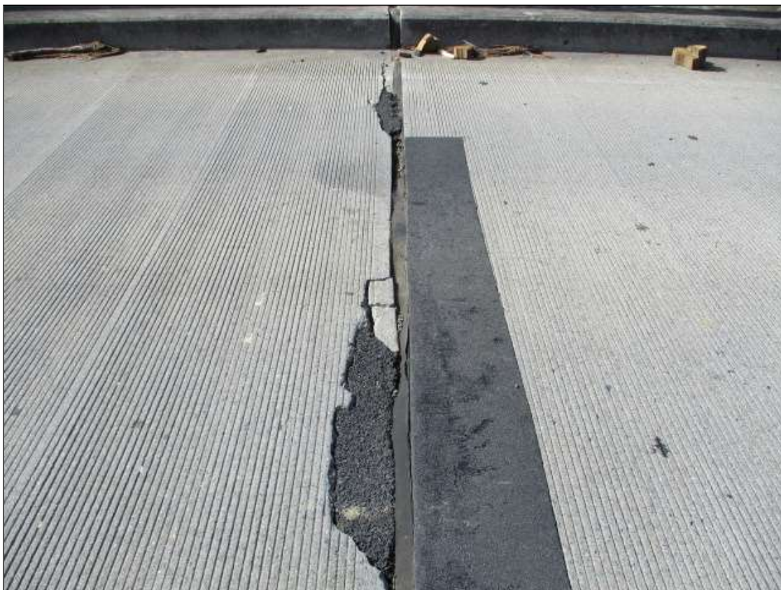
Span 26 Deck: in left shoulder AND IN SOUTH BOUND LANE at bent 26, 2 spalls [4ft x 4in x up to 2in deep]
