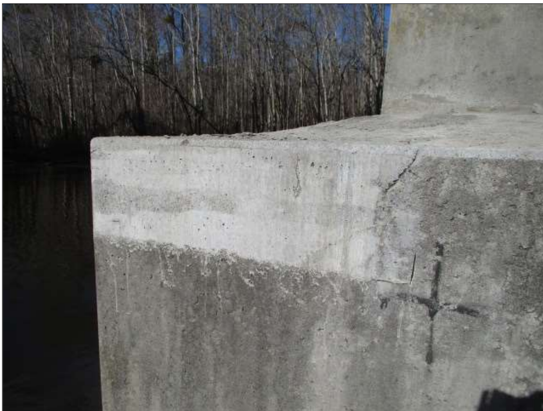
Bent 4 Footing: Northwest and Southwest corners, multiple sound patches [up to 3ft x 1ft]
