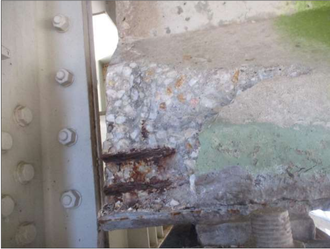
Span 20 Beam 3: PAR: SPAN 20 BEAM 3 RIGHT BOTTOM FLANGE OVER BENT 19. HAS A SPALL WITH EXPOSED STRANDS 12" LONG X 8" TALL X 3" DEEP
