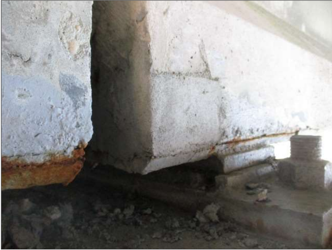
Span 61 Beam 2: 4" LONG X 4" TALL NEW REPAIR TO BOTTOM LEFT FLANGE AT BENT 61
