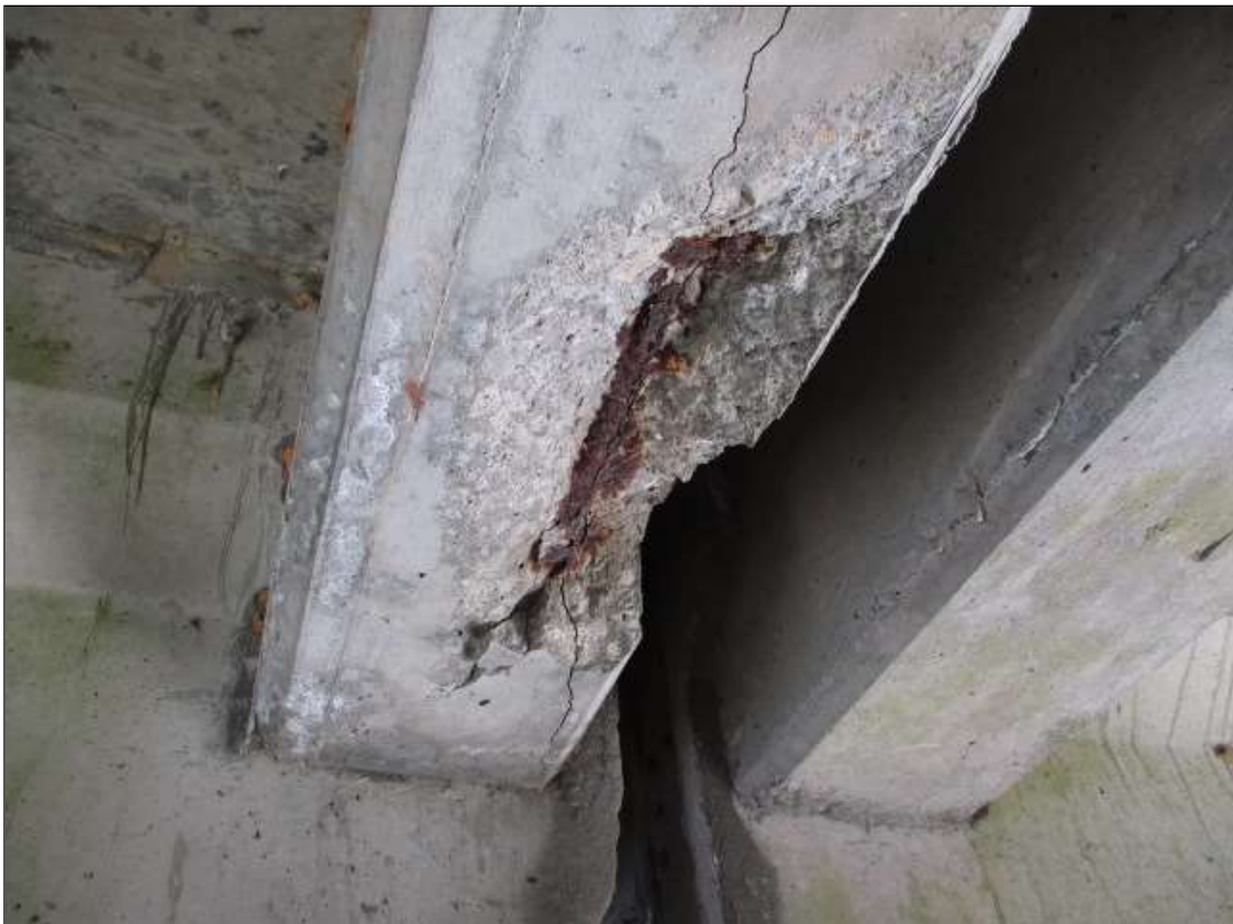
Span 13 Deck: 18" LONG X 6" X TALL X 6" WIDE SPALL WITH EXPOSED REBAR IN BAY 1 DIAPHRAGM AT BENT
