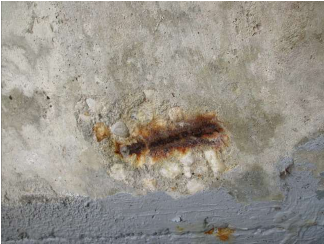
Span 23 Beam 3: underside of bottom flange at bent 23, spall [4in x 2in x 1in deep] with exposed rusted reinforcing [up to 10% section loss]
