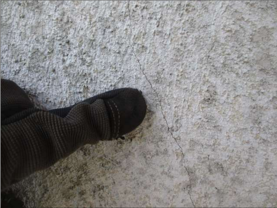
Bent 2 Pile 2: along East face, sound patch [up to 6ft x up to full width] WITH 1/32" VERTICAL CRACKING
